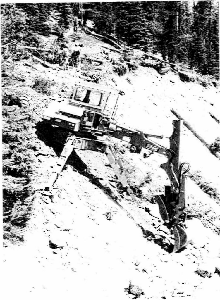
Photo 6 - Machine called a walking excavator used for initial experimentation of scaling on slopes. The slopes were found to be too steep to operate this machine safely.
