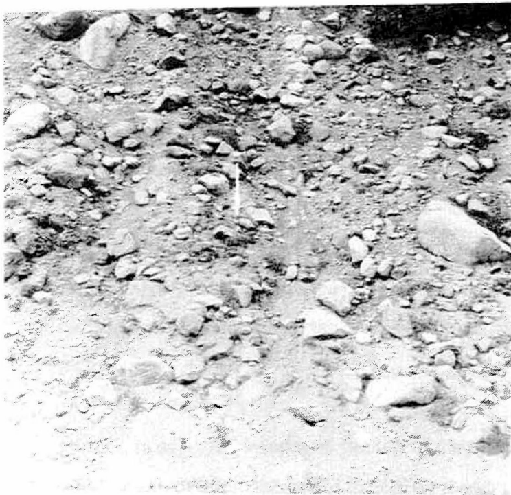
Photo 4 - Typical slope requiring scaling.
