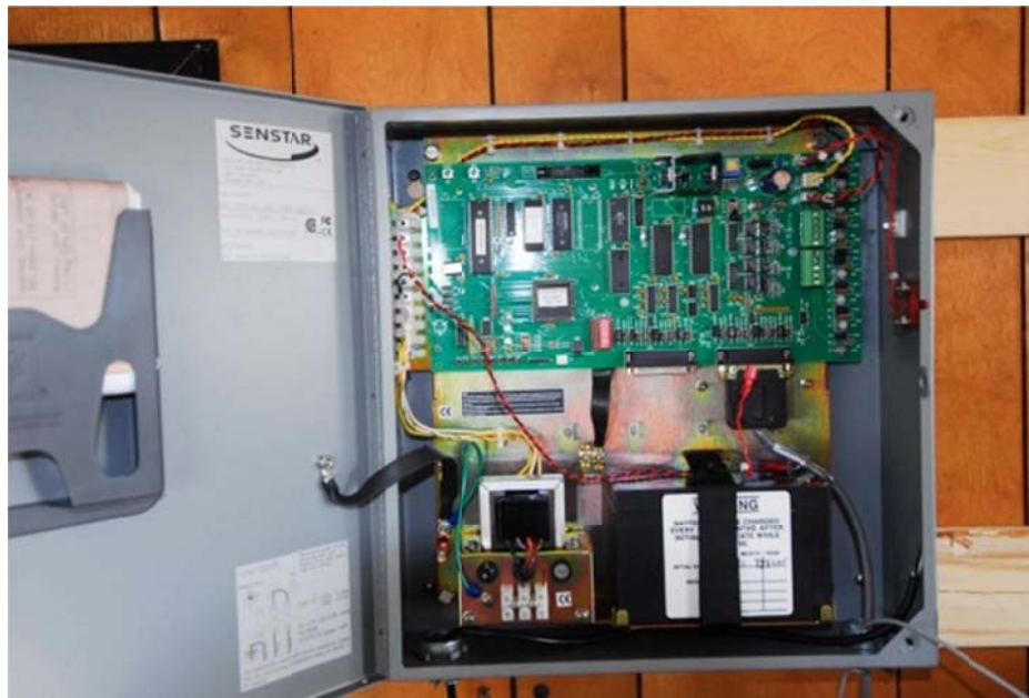
Figure 4.8: The Senstar Perimitrax® Network Controller inside the research trailer (Photo: Marcel Huijser, WTI/MSU).
