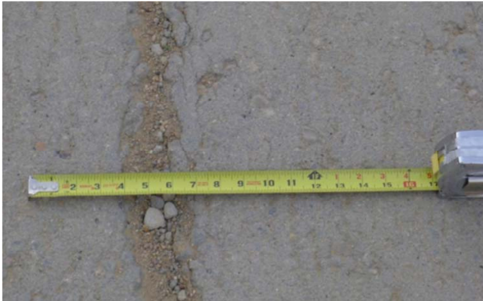
Fig. 3.9 The width of large crack on the surface of pavement at WCR 28
