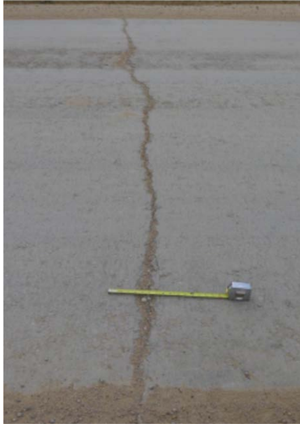
Fig. 3.8 A large crack occurs on the surface of pavement at WCR 28
