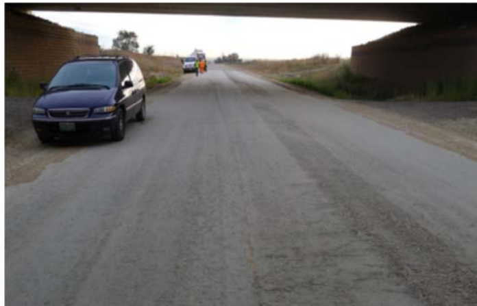
Fig. 3.1 Surface texture at WCR 28
