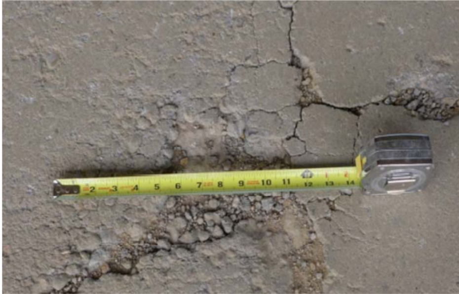
Fig. 3.10 Chipping of the pavement at WCR 28
