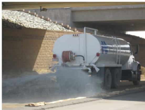
Fig. 1.2 A water truck is used for providing moisture to the base course
