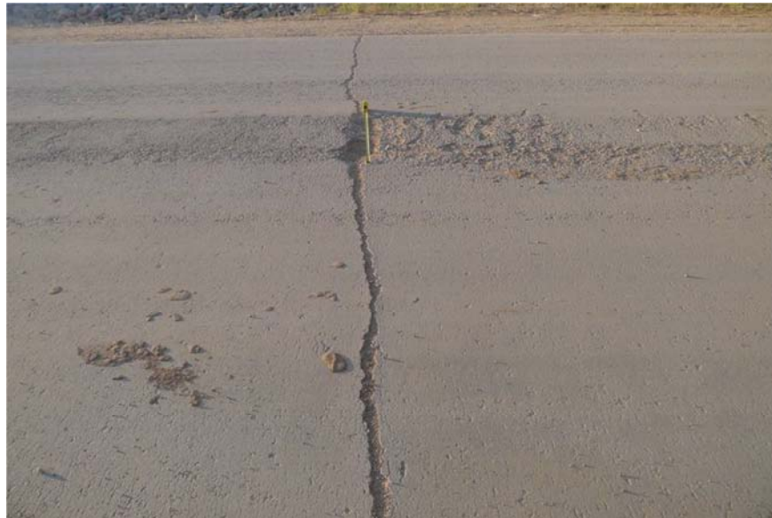
Fig. 3.17 A large transverse crack on the pavement at WCR 28 (Two years after construction)
