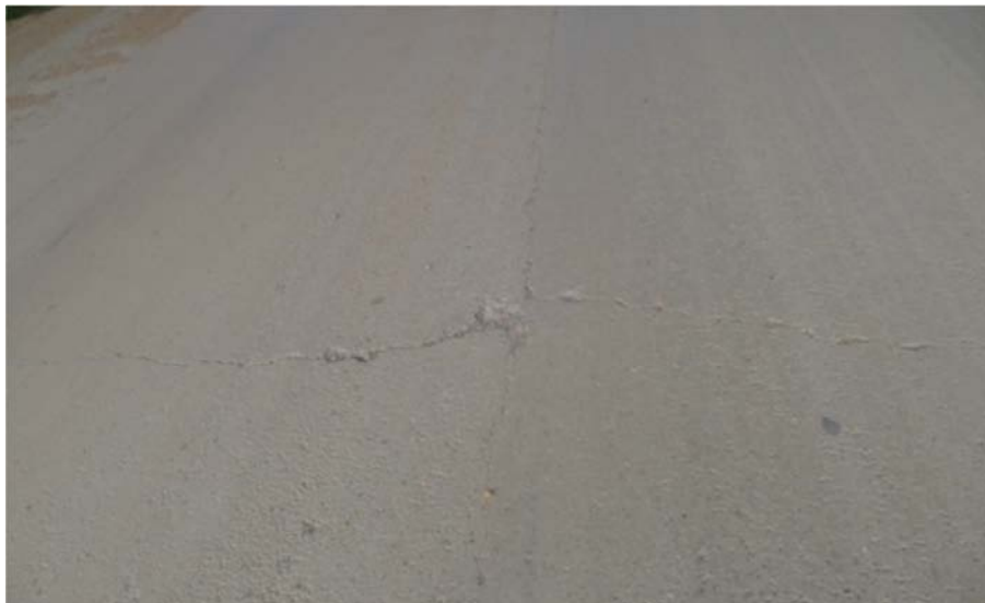
Fig. 3.6 The transverse cracks on the pavement at WCR 28
