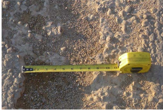
Fig. 3.18 The width of the transverse crack increased (Two years after construction)
