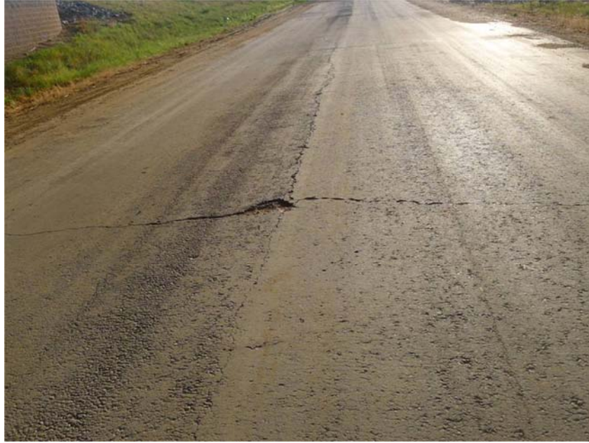
Fig. 3.16 Transverse cracks on the pavement at WCR 28 (Two years after construction)
