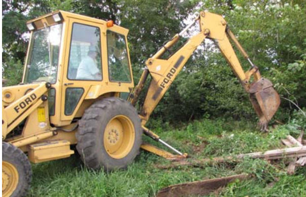
Figure 15. “Farmer John” Ellis starting hole for soil testing. This same rig will be used for digging trenches for the footer and foundation.
