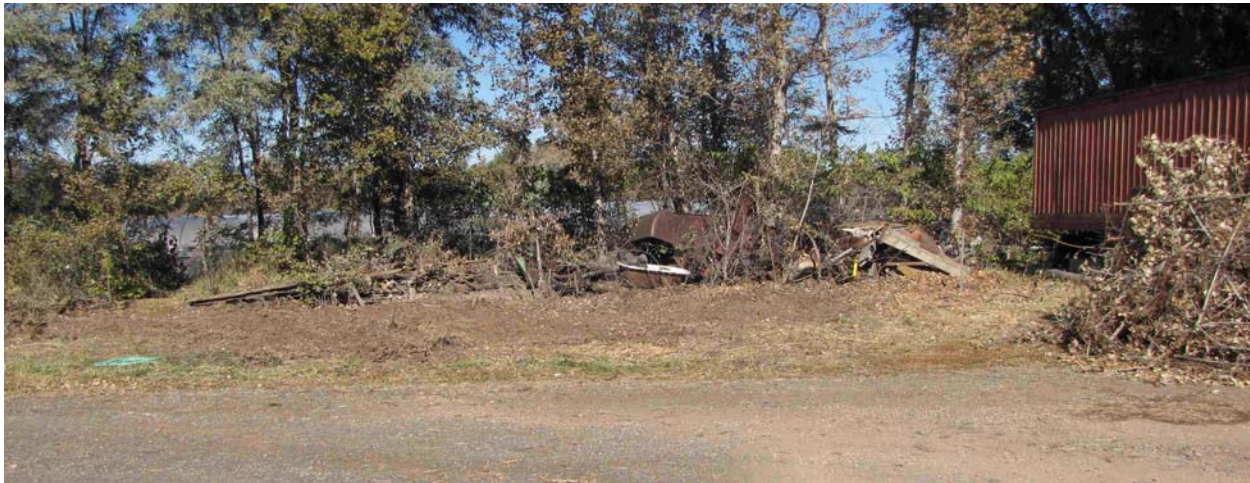
Figure 17. Site preparation nearly complete, looking north, dirt road in foreground. The greenhouse will be close to the road with its long (50 foot) axis running east and west (left to right in the photo), its short (20 feet) axis running north and south. The irrigation ditch runs between the trees.
