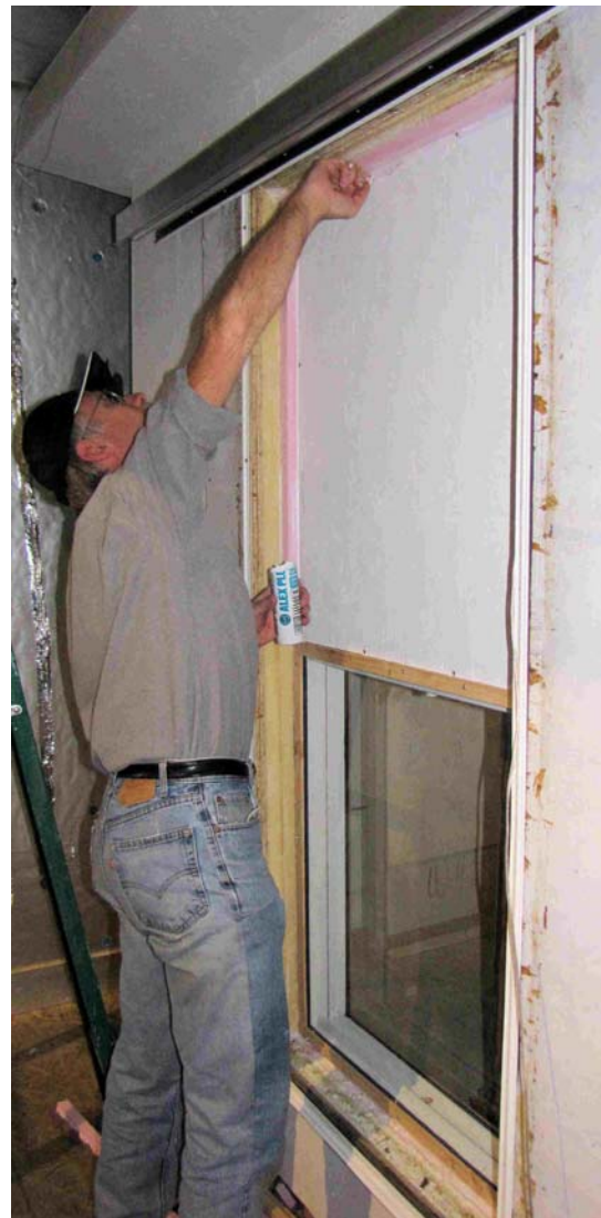
Figure 14. System being installed (and air sealed) in window testing lab, shutter in pocket.
