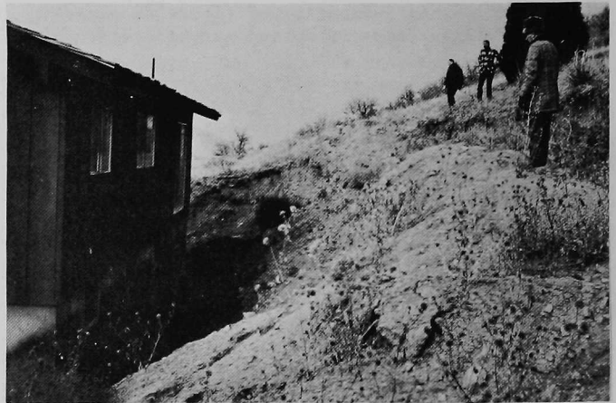
FIGURE 7. The excavation for this house foundation was made in unstable colluvium. The material on which the man in the foreground is standing has slid downslope and is causing distress in the rigid concrete foundation walls.
