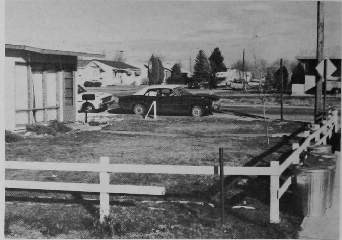
FIGURE 10. Subsidence over Strathmore mine, South Longmont Street, Lafayette. The low sag in the front lawn and the front walk are subsidence related. This "subsidence" is actually the result of compaction of trash and rubble used to fill a true subsidence pit which formed in 1956 ( Denver Post , May 27, 1956). There was rapid collapse and overnight development of a hole 40 ft deep and 15 to 20 ft square.
