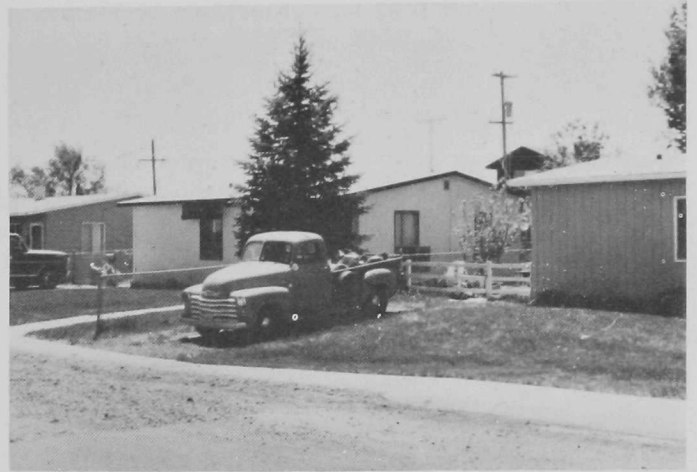
FIGURE 8. Subsidence over Strathmore mine, South Longmont Street, Lafayette. The most recent damage to the street has not yet been fully repaired. Note unpaved section of street and sagging sidewalk. The coal seam in this area of the Strathmore mine was quite thick, and the probable thickness of coal extracted was 20 to 25 ft. Depth of mining was 100 to 125 ft.
