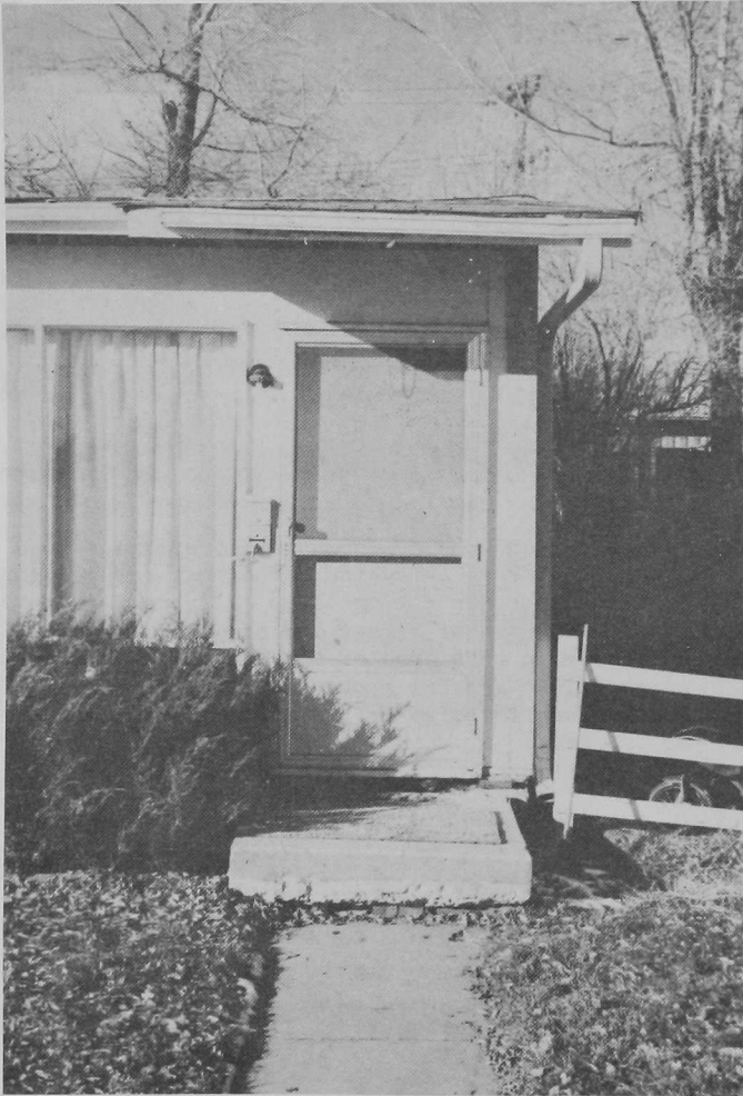
FIGURE 9. Front stoop of house to the right in Figure 8. This house is immediately south of home shown in Figure 10. The walk was pulled away from the stoop and it in turn has pulled away from the house. Bricks have been jammed beneath the house and beneath the stoop for temporary support.
