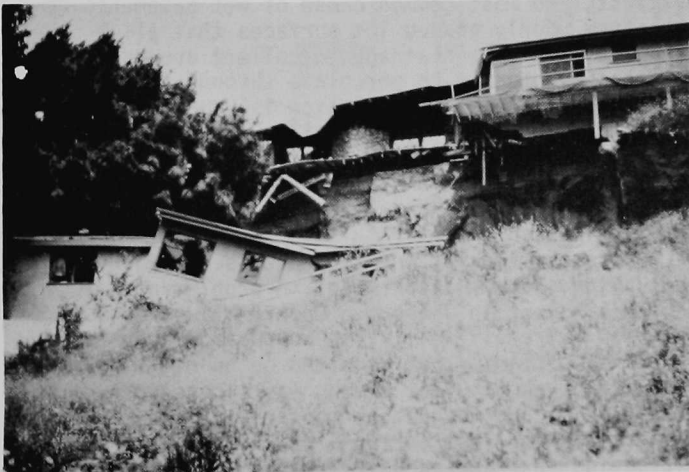
FIGURE 1. Landslide damage resulting from ground water seepage into highly fractured shale.
