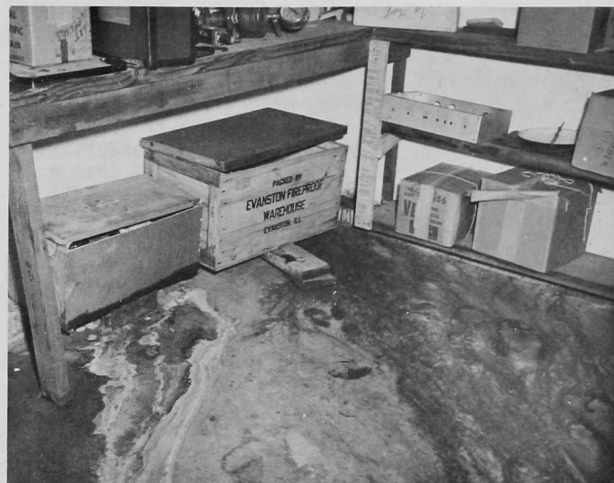
Figure 3. Water seepage flowing across basement floor in a Lookout Mountain area home near Golden, Colorado. The home is founded on crystalline rocks.
