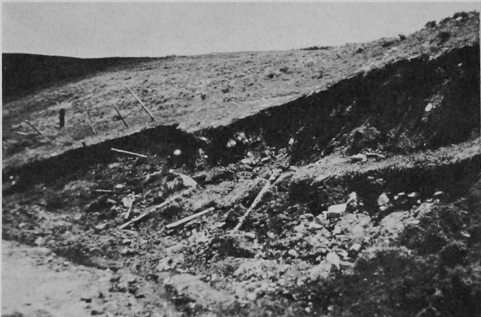
FIGURE 5. This failure of a roadcut resulted from oversteepening unstable slope-forming materials.
