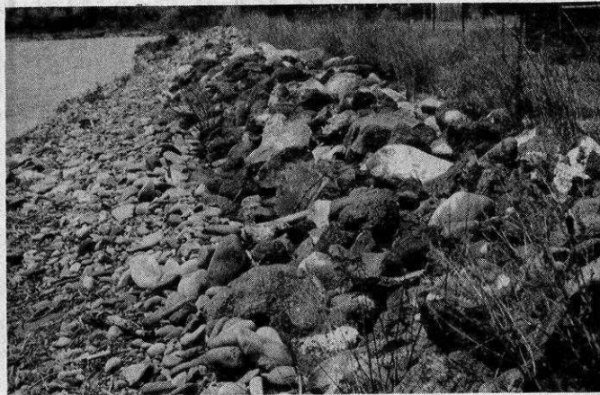
Rock Riprap protecting sewer plant on North Fork Gunnison River Photography by Jim Thornton, SCS, Denver, Colorado
