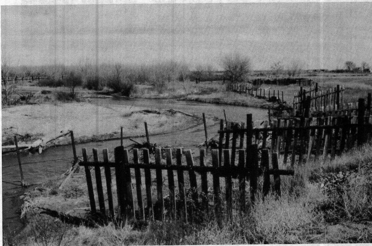
Plank jetties on Fountain Creek protecting a high pressure gasline and cropland
