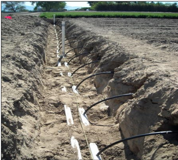
Fig. 2. Two subsurface drip zones with flush valves and drip lines exiting the main lines at the Colorado State University Western Colorado Research Center at Fruita.
