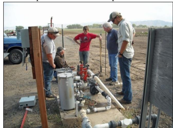
Fig. 3. Pumping and filter station for the subsurface drip irrigation system at the Colorado State University Western Colorado Research Center at Fruita.
