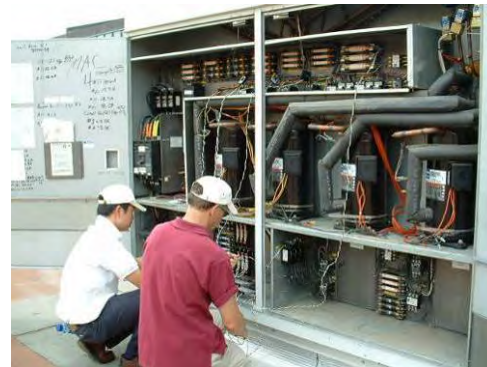
Installation of data loggers to verify performance Courtesy: Architectural Energy Corporation
