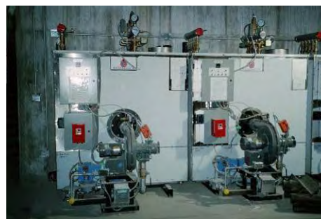
Fossil Ridge High School Condensing Boilers Time and money spent on fine-tuning the energy efficiency, yields savings because the school uses much smaller heating, cooling and electrical systems.
