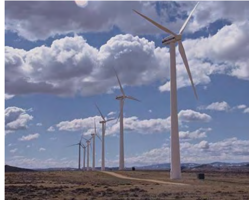
Platte River Power Authority Medicine Bow Wind Project supplies wind power to Fort Collins, Loveland, Estes Park and Longmont. Courtesy: Platte River Power Authority
