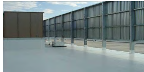
GSA Federal Department of Transportation Lakewood office building's white membrane roof Courtesy: Opus Northwest
