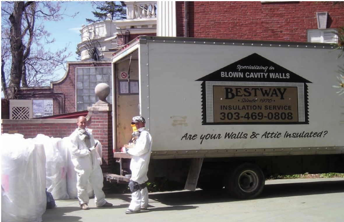
Amory Barton and Kyle Willie of Broomfield-based Bestway Insulation take a break while installing insulation at the Colorado Governor's Residence at the Boettcher Mansion in Denver.
