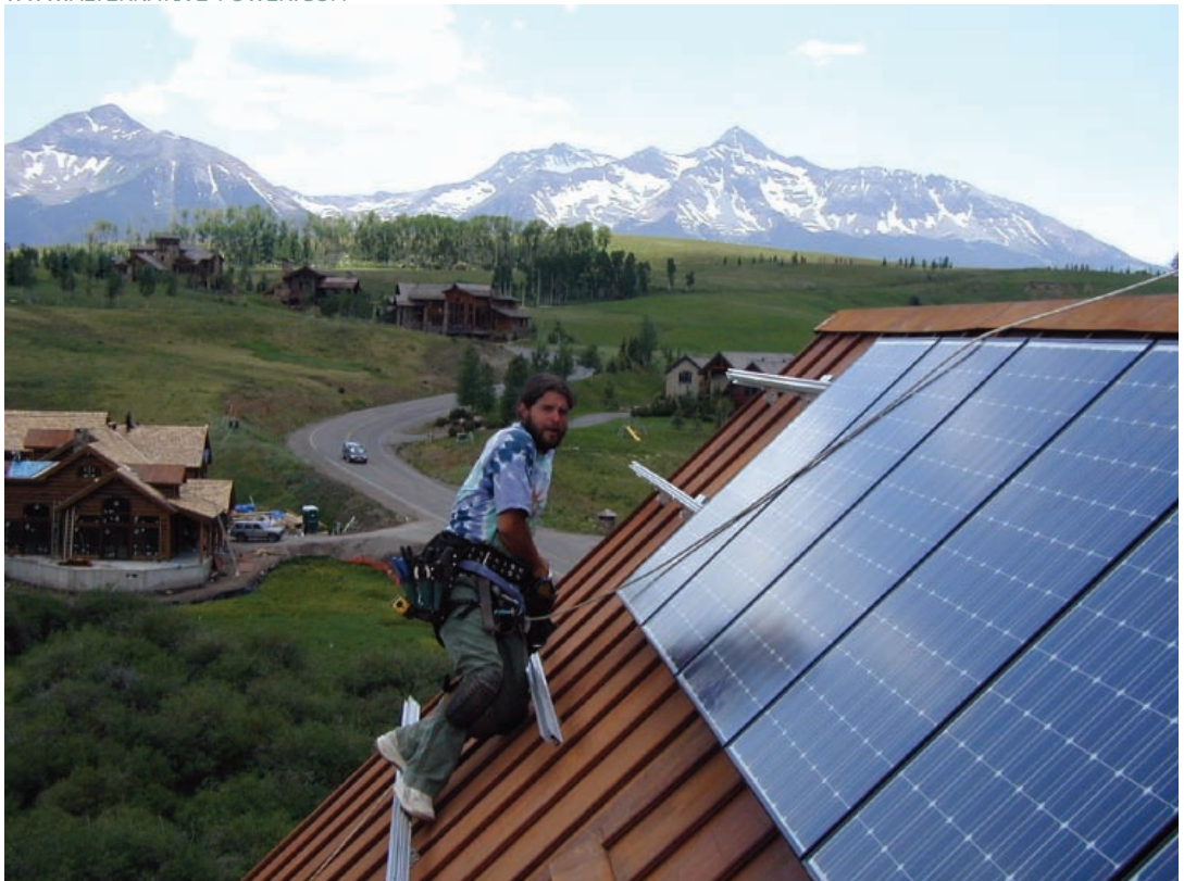
An employee of Ridgway-based Alternative Power Enterprises installs a photovoltaic system on a home in Mountain Village, Colorado, in 2007.
