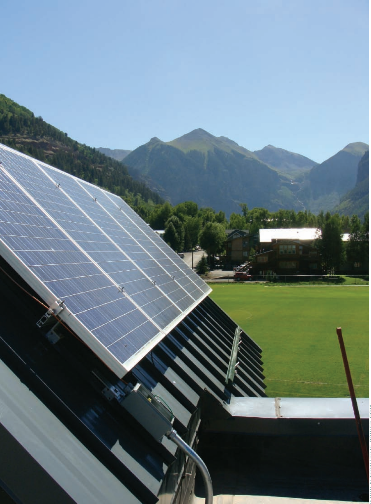
Ridgway-based Alternative Power Enterprises installed this 1.9-kilowatt photovoltaic system on Telluride High School as part of a collaborative and community demonstration project.
