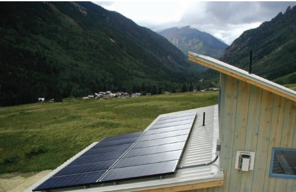
Ridgway-based Alternative Power Enterprises installed this photovoltaic system in Ophir, Colorado, in August of 2007.
