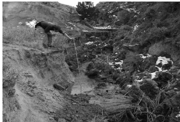
Figure 3. Erosion in Ephemeral Drainage
