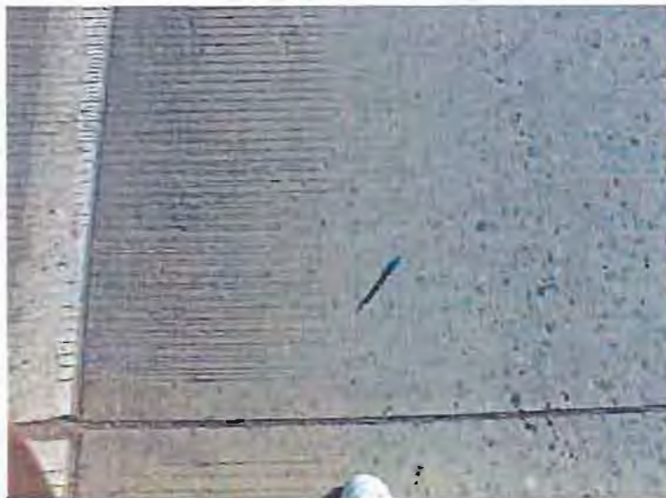
Figure 4. A detailed view of transverse tining at Test Section 1 between mileposts 244.42 and 244.45, east-bound US285. The right-hand ½ of the photograph shows where transverse tining has been ground. The grinding tapers to the left showing remnant transverse tining texture. Note pen for scale.
