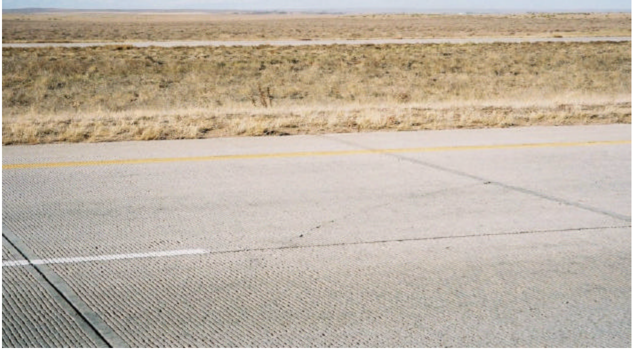
Figure B-11. Occasional Slab Crack on I-76 (Eastern Site).
