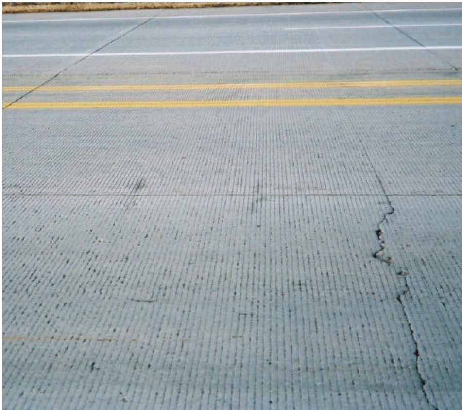
Figure B-16. Mid-Panel Crack and Tie-Bar "Scarring" on US-34.
