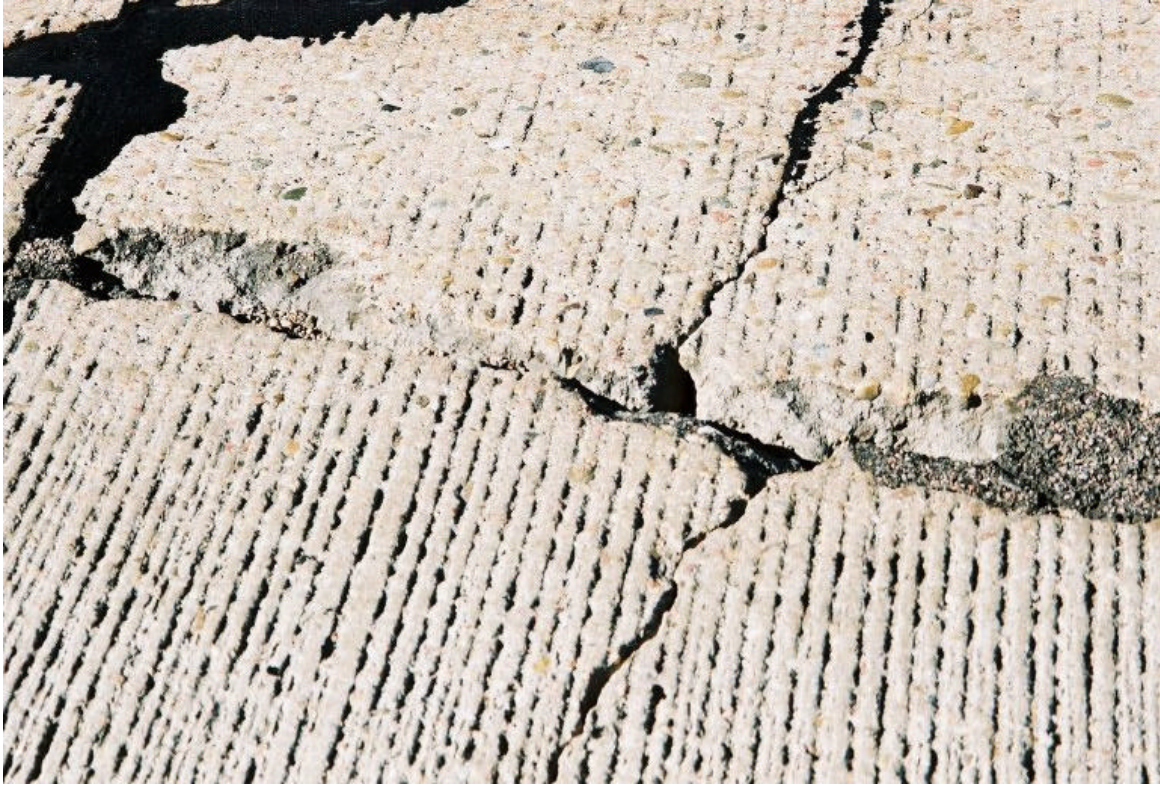
Figure B-7. Severe Spalling on I-76 (Western Site).
