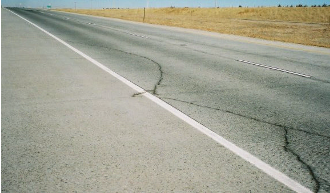
Figure B-1. Longitudinal Cracking of I-70.
