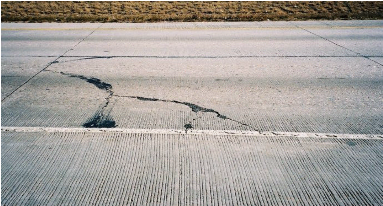
Figure B-18. Shattered Slab on I-25.
