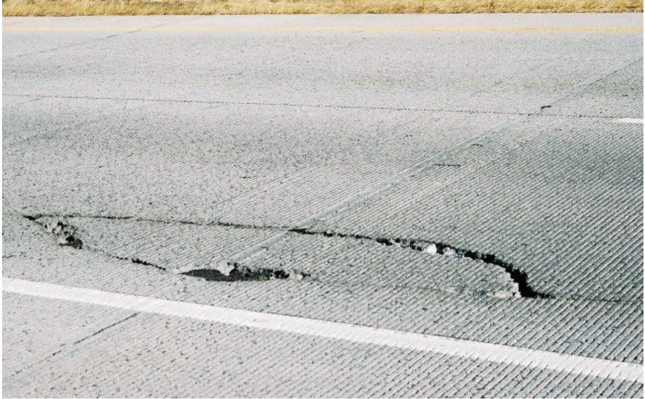
Figure B-3. High Severity Spalling of Cracks on I-70.
