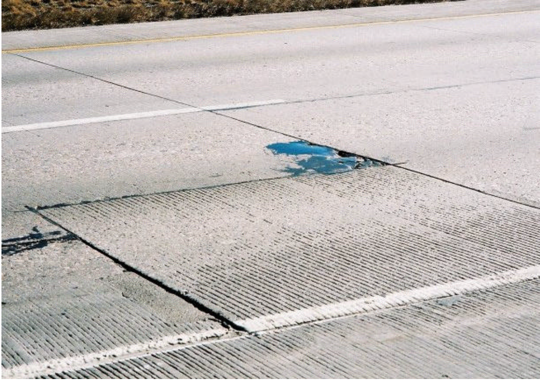
Figure B-19. Failing PCC Patch on I-25.
