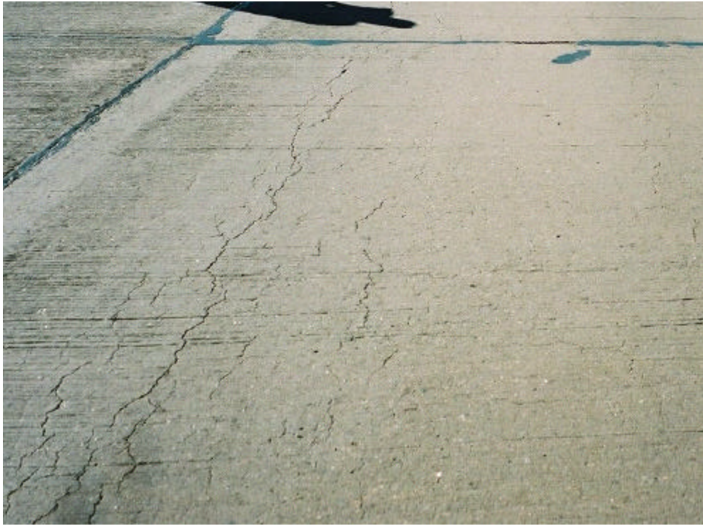
Figure B-5. Possible Fatigue Cracking on I-76 (Western Site).
