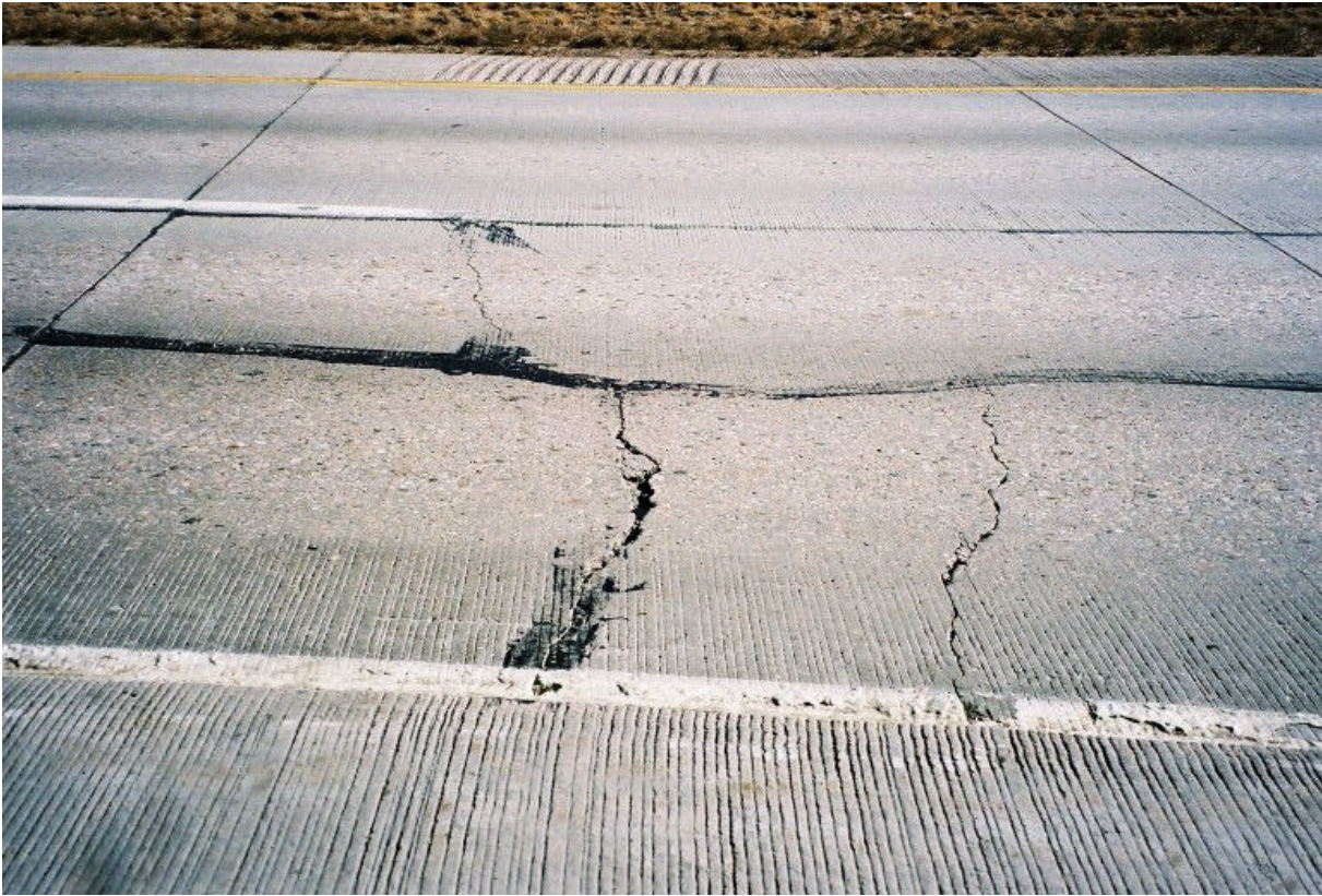
Figure B-17. Shattered Slab on I-25.
