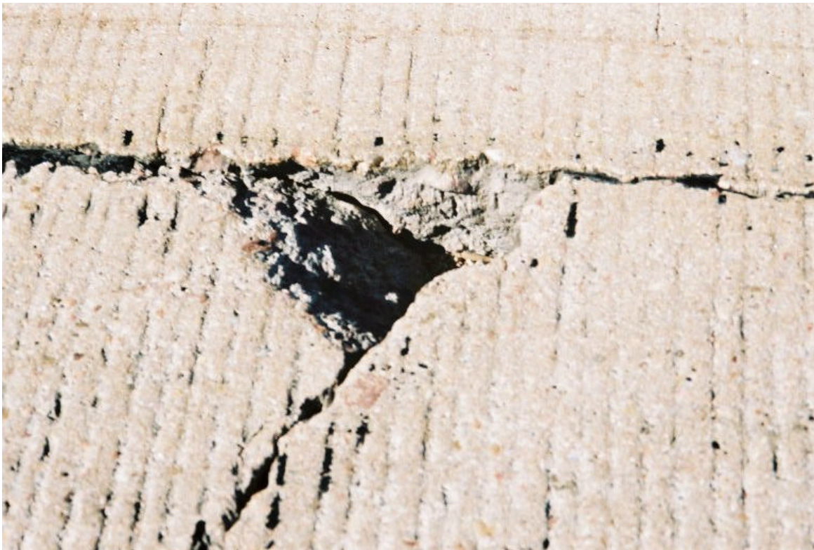
Figure B-8. Severe Spalling on I-76 (Western Site).
