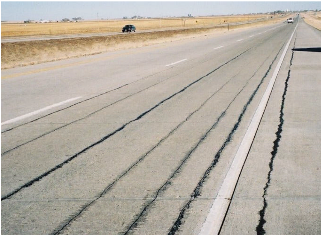
Figure B-10. Traffic Scarring of Pavement Falsely Identified as Longitudinal Cracking by PMS on I-76 (Eastern Site).
