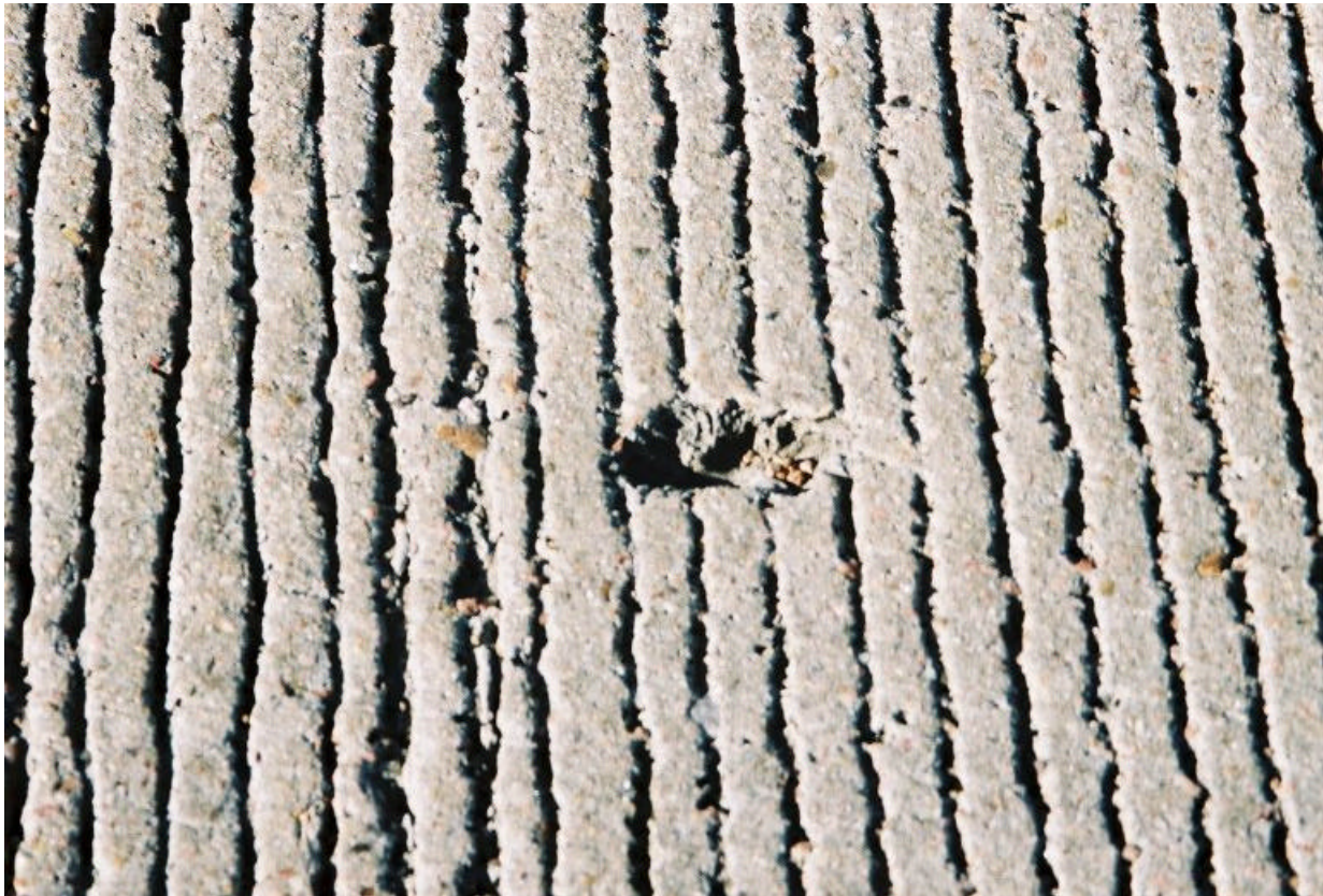
Figure B-12. Occasional Minor Popout on I-76 (Eastern Site).
