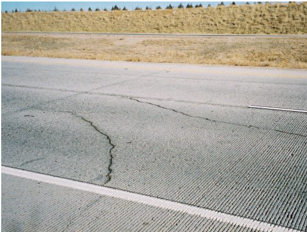
Figure B-2. Longitudinal Cracking of I-70.
