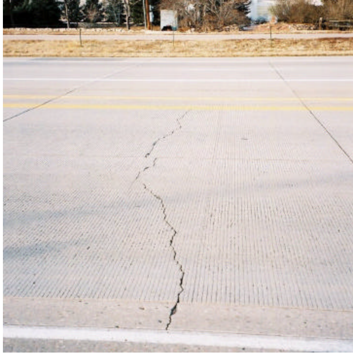
Figure B-15. Localized Mid-Panel Transverse Cracking on US-34.
