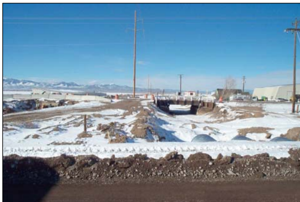
Figure 1.3. Detour drainage structure. Prairie Bridge and 60-inch pipes (CDOT Region 5).
