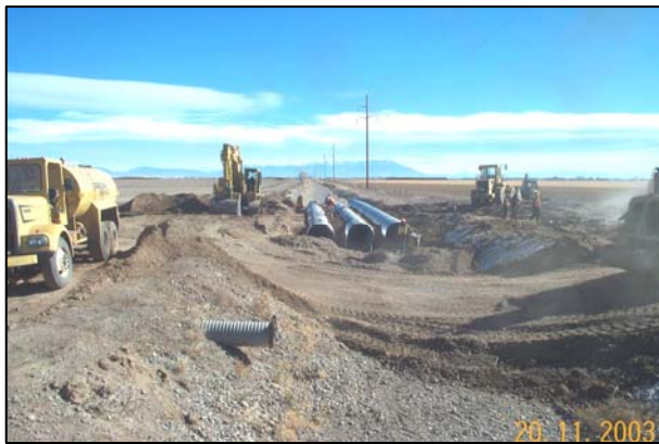
Figure 1.1 Construction of detour drainage structure. Three 60-inch pipes in Prairie Ditch under detour (CDOT Region 5).
