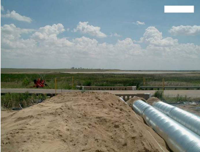
Figure 3.2. Construction of detour culverts on US Highway 50 by John Martin Reservoir in CDOT Region 2 within environmentally sensitive areas.
