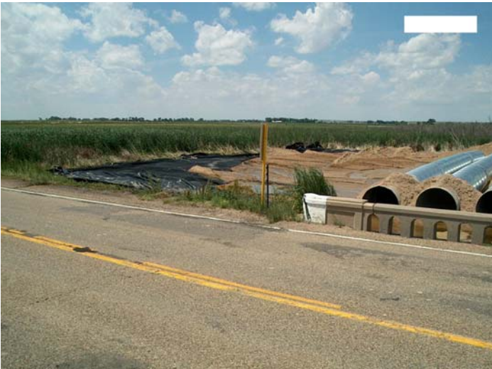
Figure 3.3 Use of geotextiles for the temporary protection of wetlands during construction of detour culverts on US Highway 50 by John Martin Reservoir in CDOT Region 2.
