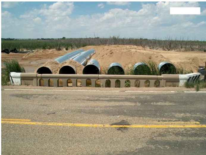
Figure 3.4. Construction of detour culverts within environmentally sensitive areas on US Highway 50 by John Martin Reservoir in CDOT Region 2.
