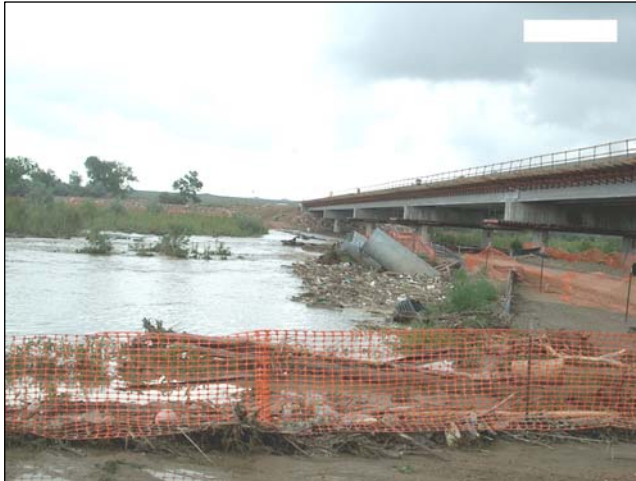
Figure 1.4. View of failed Pinon Bridge detour drainage structures on Fountain Creek. Spring 2004 (CDOT Region 2).
