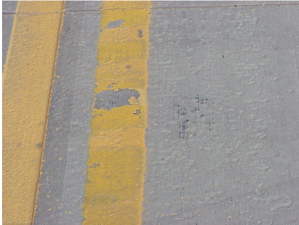
Figure 8. Epoxy paint in a groove in perfect condition next to damaged paint on the surface.
