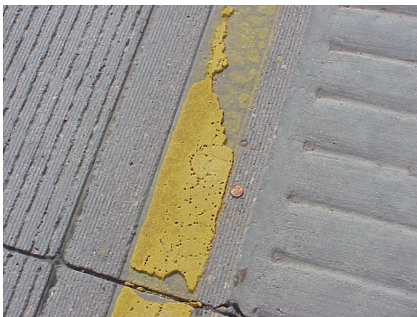
Figure 7. The thermoplastic failed due to adhesion loss.
