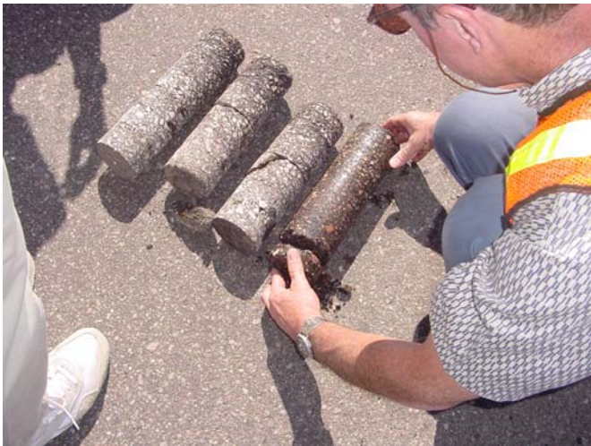
Figure 21 - It is apparent from this picture that the stripping occurs only immediately at the joint. Only the core sample right over the construction joint (right core) has evidence of stripping.
