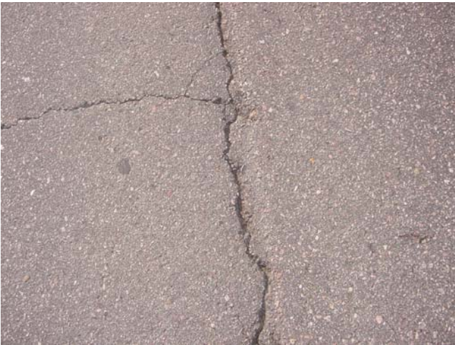
Figure 15 - Close-up view of a fairly open construction joint crack.
