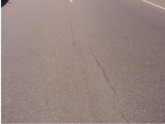
Figure 22 - This photo shows an offset crack from the construction joint, possibly the reflective crack from the original construction joint.
