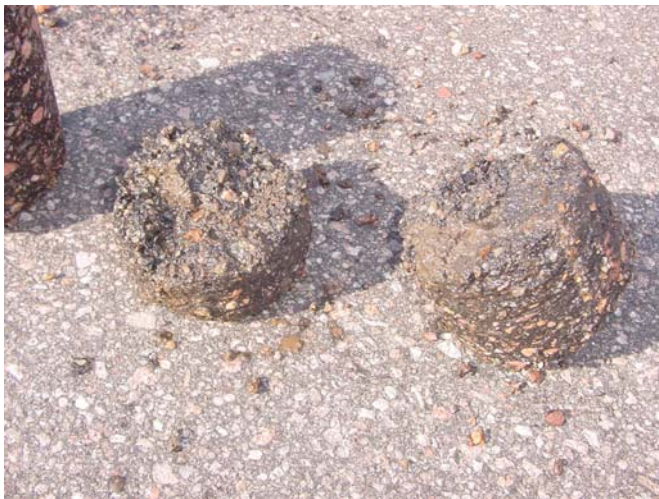
Figure 19 - Fragmented and badly stripped cores .
