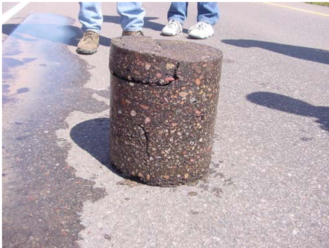
Figure 23 -The resulting core verifies the crack propagation is emanating from the underlying existing pavement layer.
