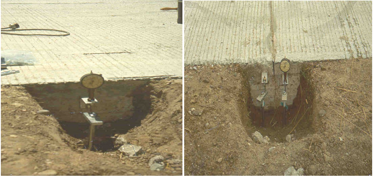
Figures 17 and 18: Acquisition of Curl Data at Mid-Slab and Corners Using Dial Gauges
