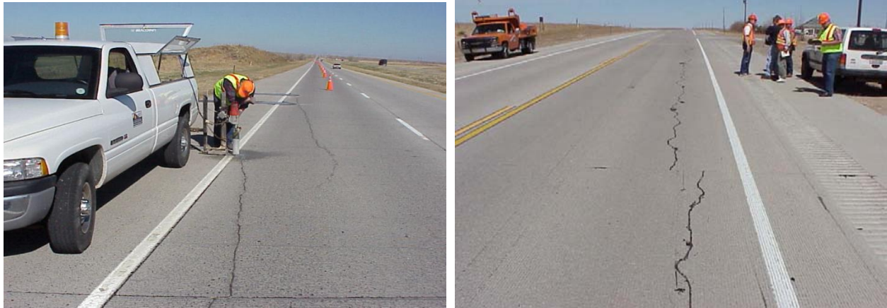
Figures 22 and 23: Longitudinal Cracks Due to Improper Depth of Saw Cut
