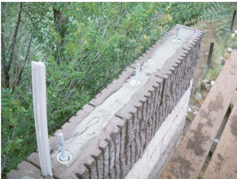
Figure 9. View of the top of the post-tensioned wall showing the sleeve inserted into the bond beam to prevent bonding of the tendon. Mortar beds were placed beneath the bearing plates to form the anchorage at this course. An additional ungrouted course was placed above the anchorage and the wall was topped with a precast concrete cap.
