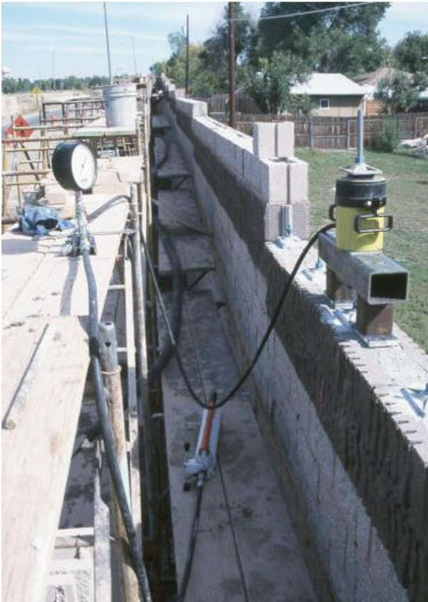
Figure 5. A hand hydraulic pump was used with a hydraulic ram to accurately tension the instrumented and intermediate tendons.
