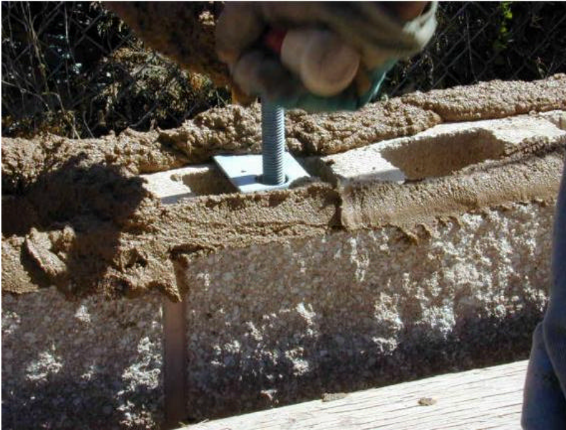
Figure 7. Photograph of the wall under construction. A tendon restraint plate can be seen in the center of the photograph.
