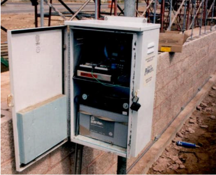
Figure 8. View of the instrument cabinet and the partially built post-tensioned wall in the background.
