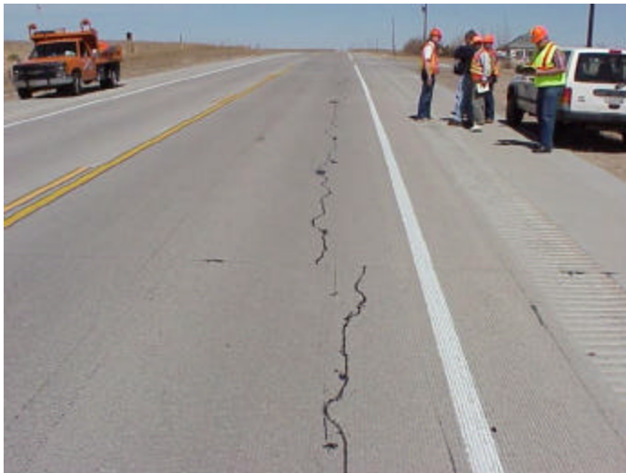
Figure 7. Wandering cracks in the northbound lane of US-287.
