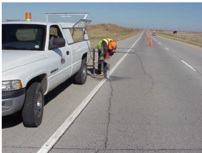
Figure 8. Longitudinal cracks on 12' wide slabs - I-70 at Deer Trail.
