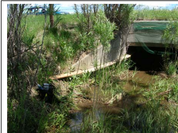
Goodhue Ditch at U.S. 36. Ramp is long and vegetation is well-developed; ledge not visible inside culvert. Note green netting for birds.
