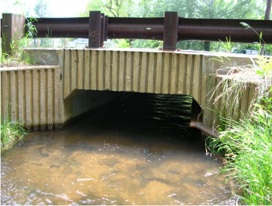
Culvert 5. Marshallville Ditch at Marshall Road. Both ledge and ramp visible at right; note strap hinge to connect them.
