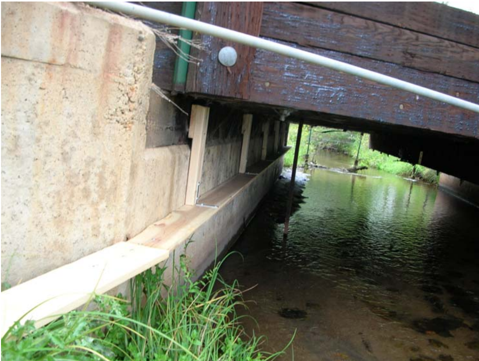
Culvert 6. South Branch of St. Vrain Creek at Crane Hollow Road. This culvert was eliminated from the study (see text). Ledge is inside culvert, ramp is on wing wall.
