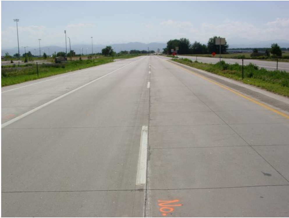
Figure 4.6. Typical Pavement Conditions Observed at the S.H. 119 Longmont Site
