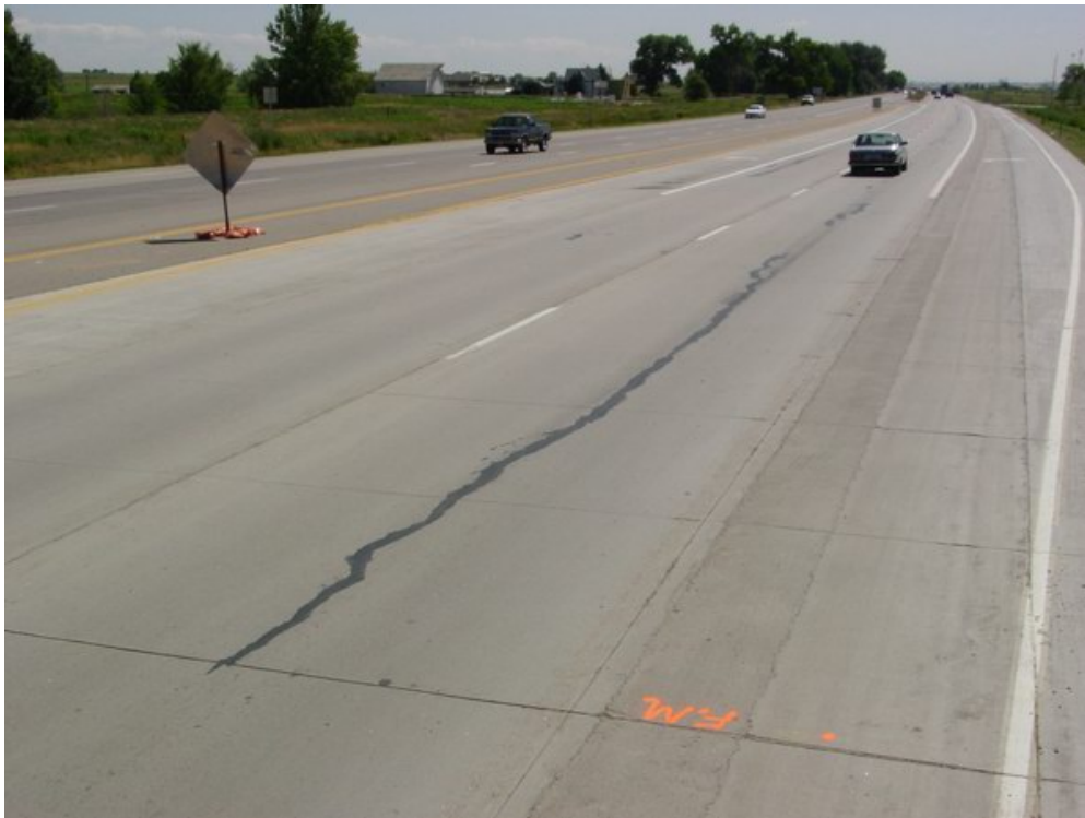
Figure 4.7. Typical Slab Cracking Observed in S.H. 119 Test Section No. 2
