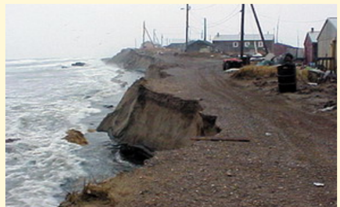
A view of damage due to permafrost melting and bluff erosion in the Alaska Native village of Shishmaref. Due to these conditions, exacerbated by climate change, the only viable option is to relocate the village. This move is expected to be completed by 2009 and could cost well over $100 million. Photo Source, NOAA.
