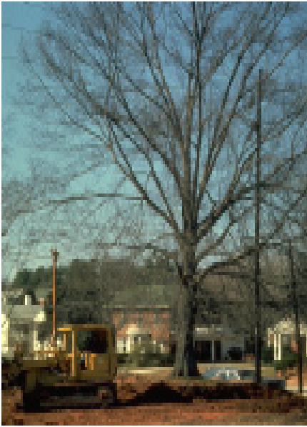
Figure 3: Root destruction, soil removal and soil compaction from construction equipment.
