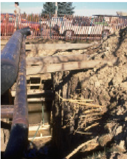
Figure 4: Trenching can severely injure a tree. Instead, auger under roots.
