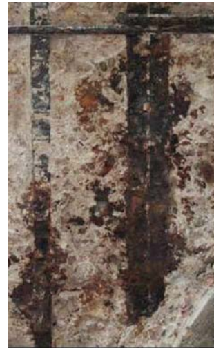
Figure 2-4 The corrosion in arch
