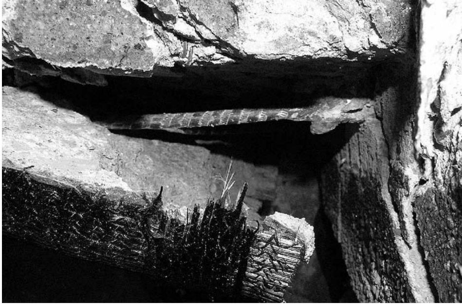
Figure 1-68 FR specimen tension Leadline between concrete and shotcrete
