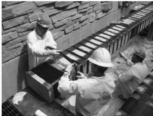
Figure 1-40 Placing final transverse wrap on AR specimen. The man below the beam is rolling more epoxy into the freshly applied wraps.
