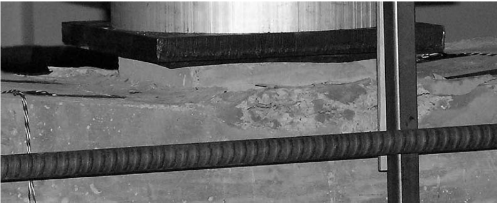
Figure 1-47 Concrete spalling around central cap (AC specimen)
