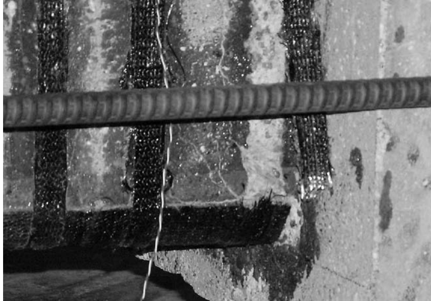
Figure 1-64 Ruptured transverse Fibrowrap where shotcrete pulled away from FR specimen
