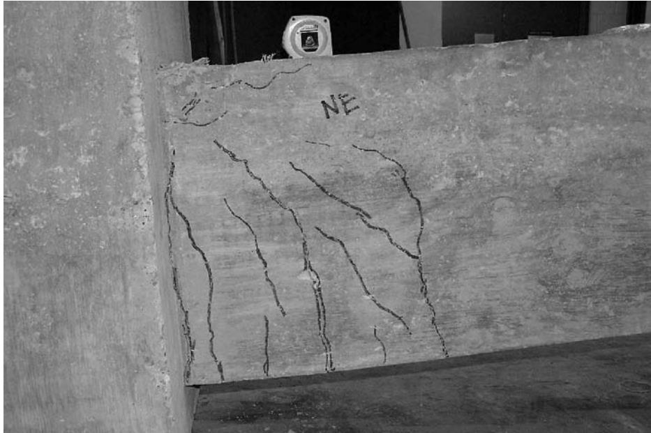
Figure 1-59 Final crack pattern at non-critical side of specimen (FC specimen)
