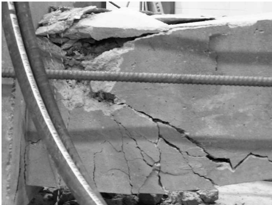
Figure 1-60 Final crack pattern at critical side of specimen (FC specimen)
