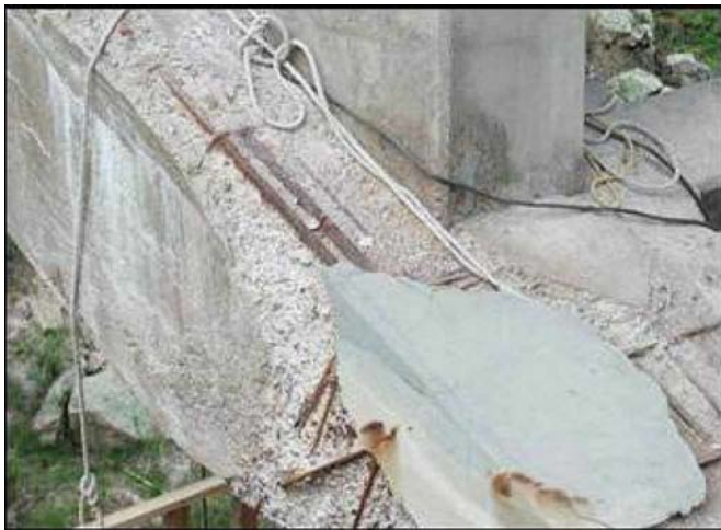
Figure 2-3 The damaged arch due to corrosion
