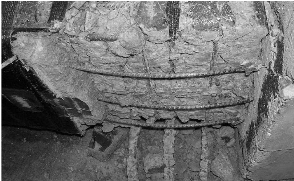
Figure 1-69 FR specimen tension Leadline with loose shotcrete patch removed
