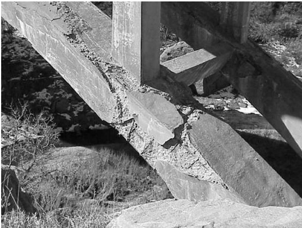
Figure 1-3 Spalling concrete and exposed steel before repair
