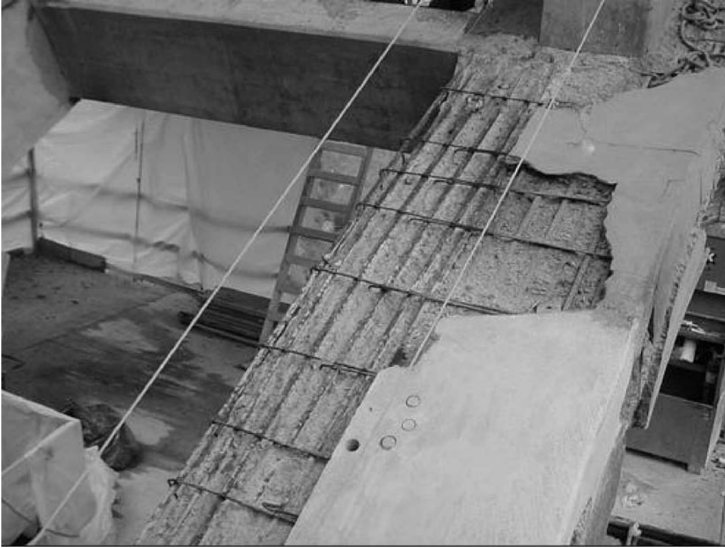
Figure 1-4 Spalling concrete and exposed steel during construction
