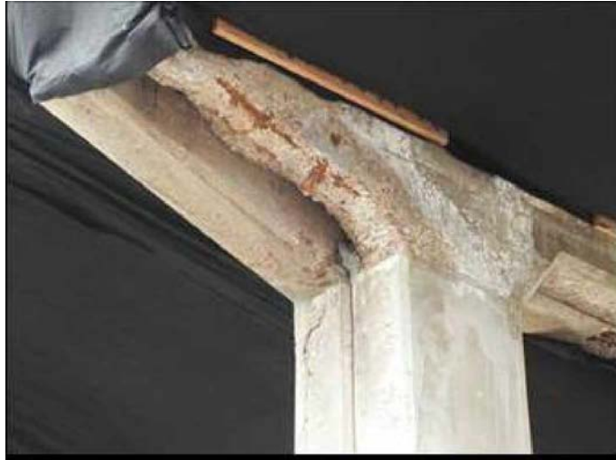
Figure 2-2 The corrosion-induced spalling in the spandrel column
