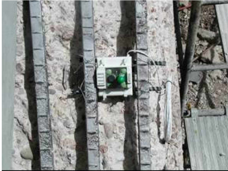
Figure 3-10 An installed corrosion sensor (ECI-1)
