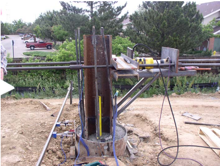
Figure 5.14 Setup of measuring devices at shaft 1 (North)
