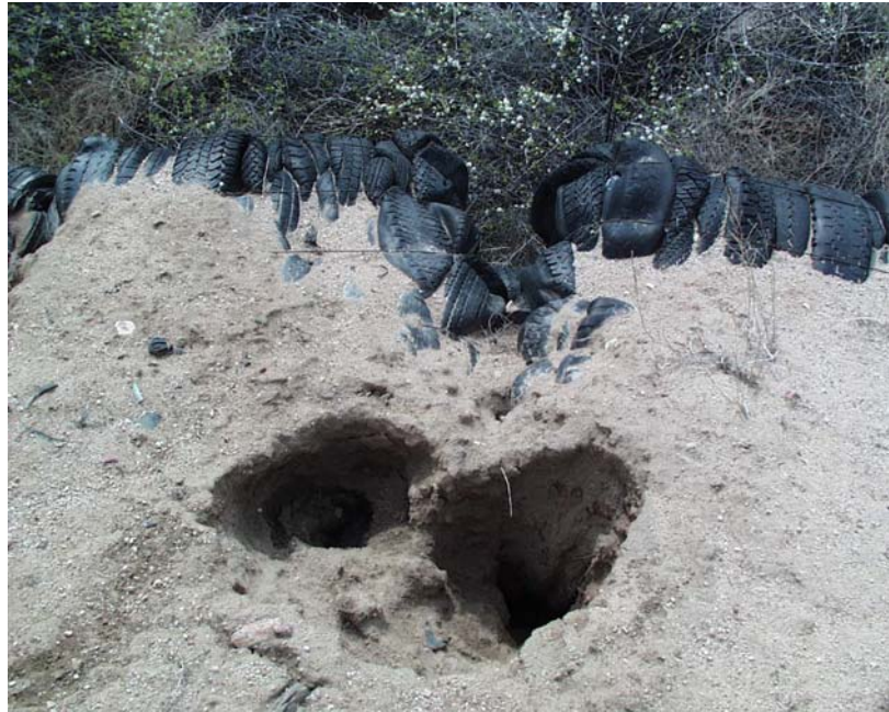
Figure B4. Typical sinkhole.
