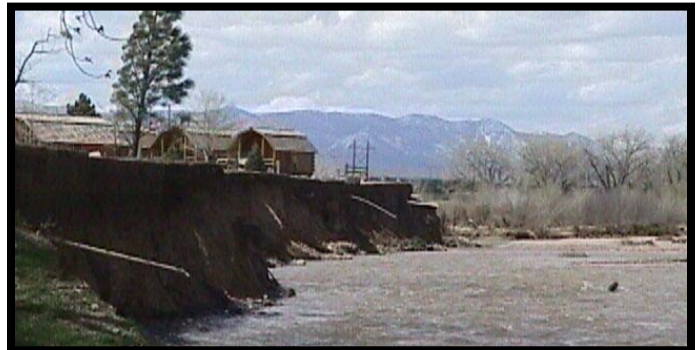
Although these structures may be outside the 100-year floodplain, it would not be prudent to develop this close to an unstable channel. Erosion buffer zones and setback limits from waterbodies preserve natural riparian function and reduce flood hazard risks.
