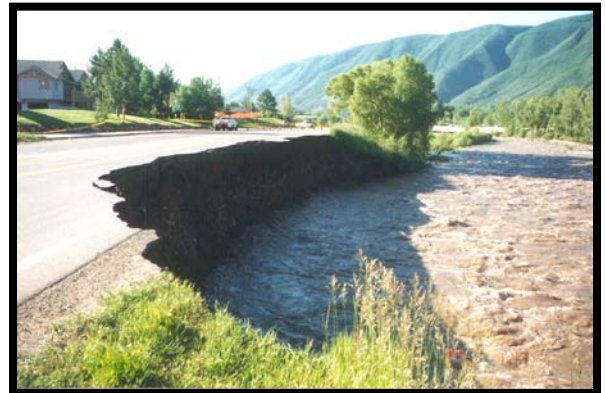
This roadway was outside the 100-year floodplain, but nonetheless, still at risk to flood hazards.
