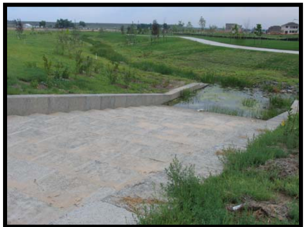
This concrete spillway safely routes emergency flows down the embankment and was landscaped to have the general appearance of a staircase.
