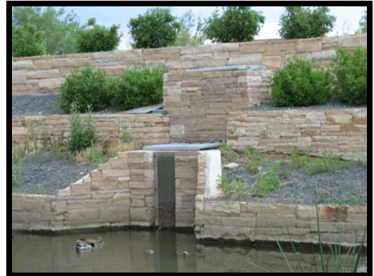
Rather than a concrete box in the middle of the pond, this outlet was effectively landscaped into the embankment.
