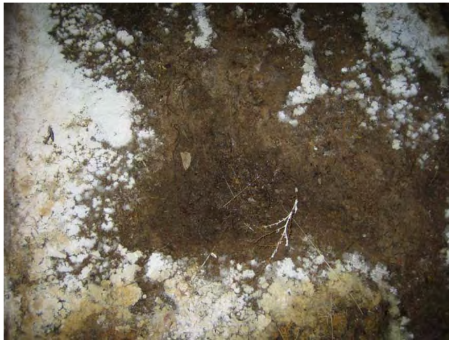
Figure 13. Concrete pipe corrosion at Site 4 (North of Walsenburg)
