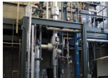
Plant B Water Deionization Unit
