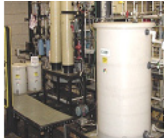
Plant A Fluid Handling
