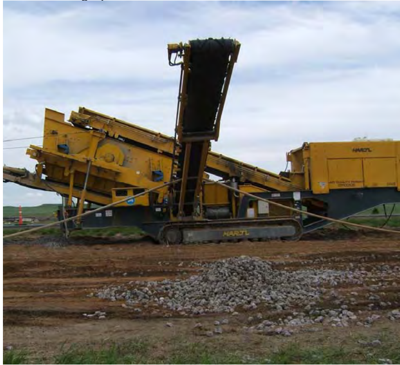
Figure 5-1 Photographs of Mobile Screen Plant
