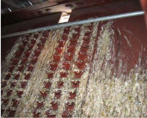
Figure 3. 3-inch gap in splice in Gir 5A (E16ND).
