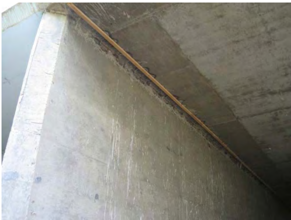
Figure 8. Lath Remaining After Removal of Plastic Strips; Blue Ceiling of Adjacent CBC Visible in Left of Photo.
