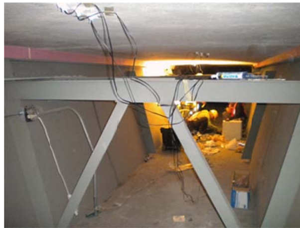
Fig 3.15 Sensor wiring from inside of the steel box girder
