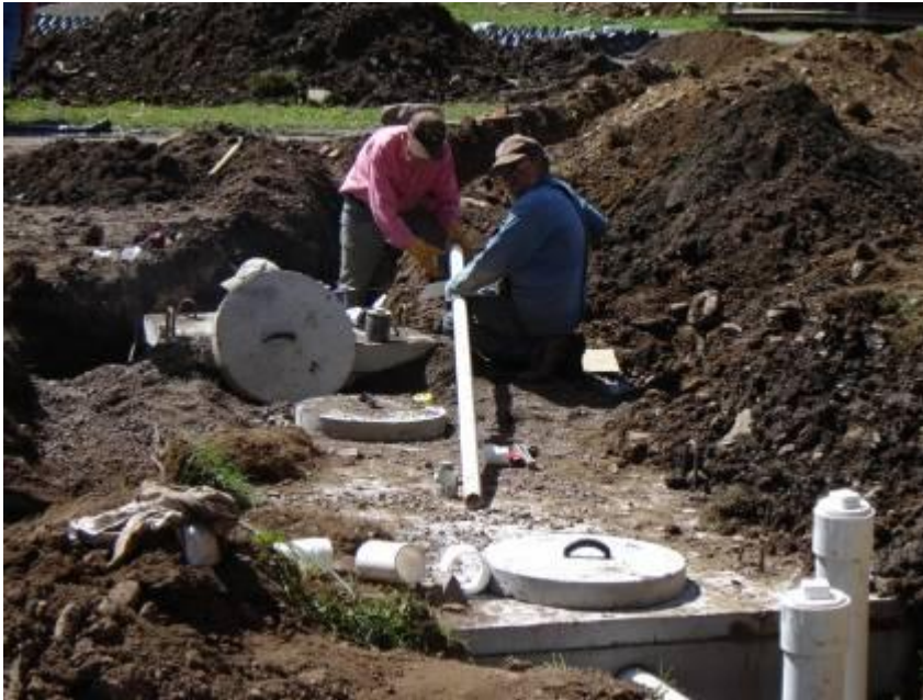
Figure 9. The Lodge's Septic Tank Installation in 2007 (Source: Conejos County Land Use office)
