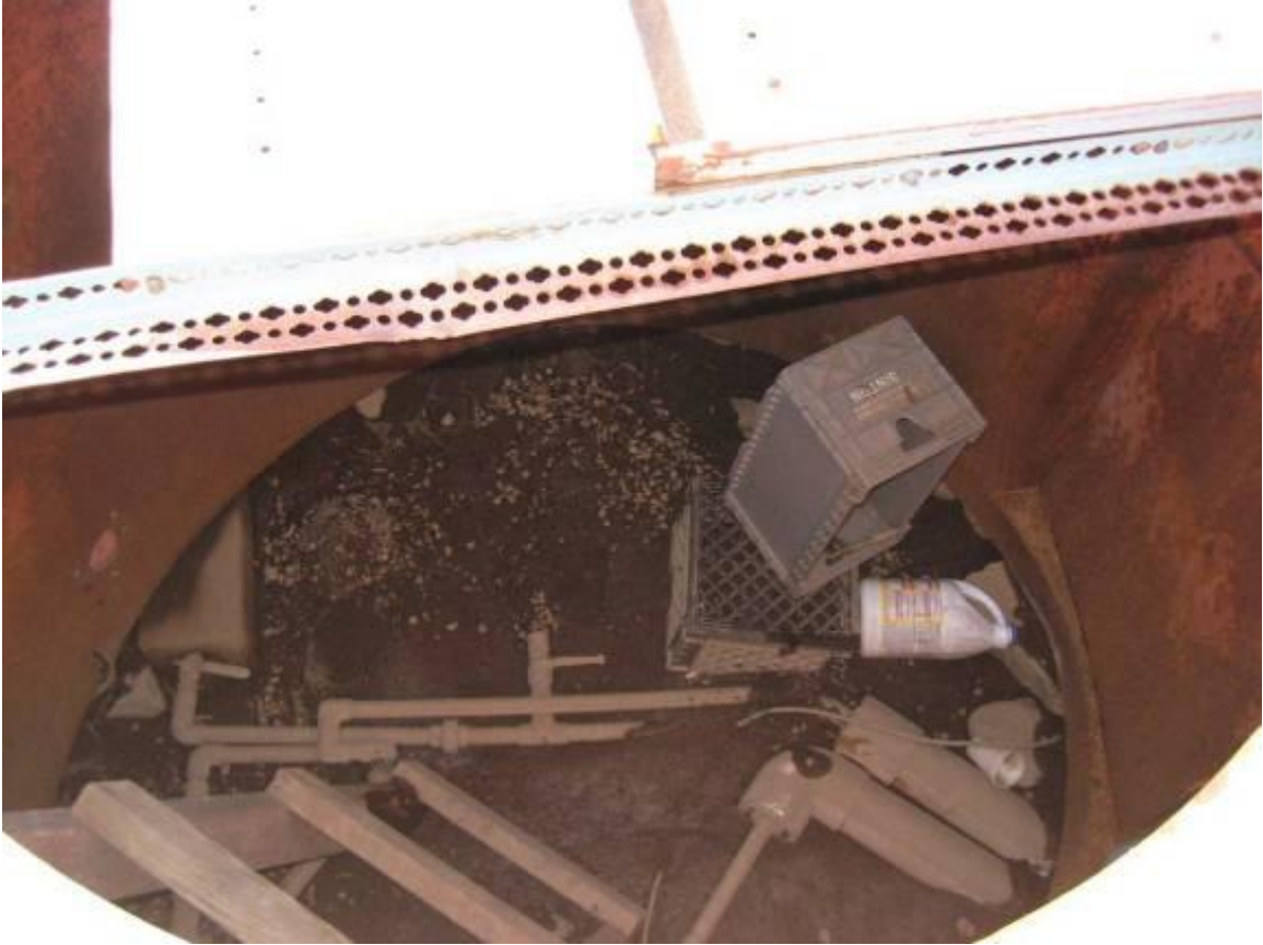
Figure 7. Abandoned Well Observed During the 2010 Sanitary Survey
