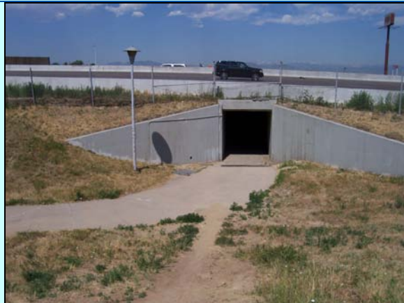
Photo 5-2: 120th Avenue Transit Station Underpass facing west, on the east side of I-25.
