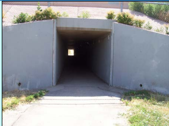
Photo 5-1: 120th Avenue Transit Station Underpass, facing east from the west side of I-25.
