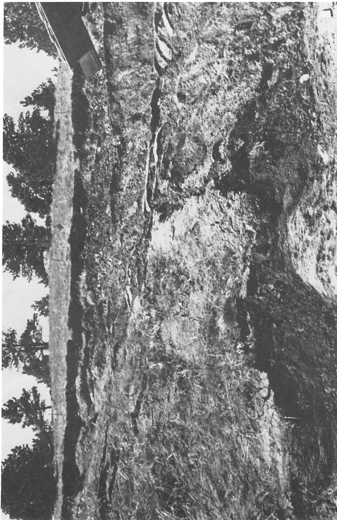
Figure 29. What had been a slope in equilibrium is now a geologic hazard because of human activities (photo by J. A. Pendleton).
