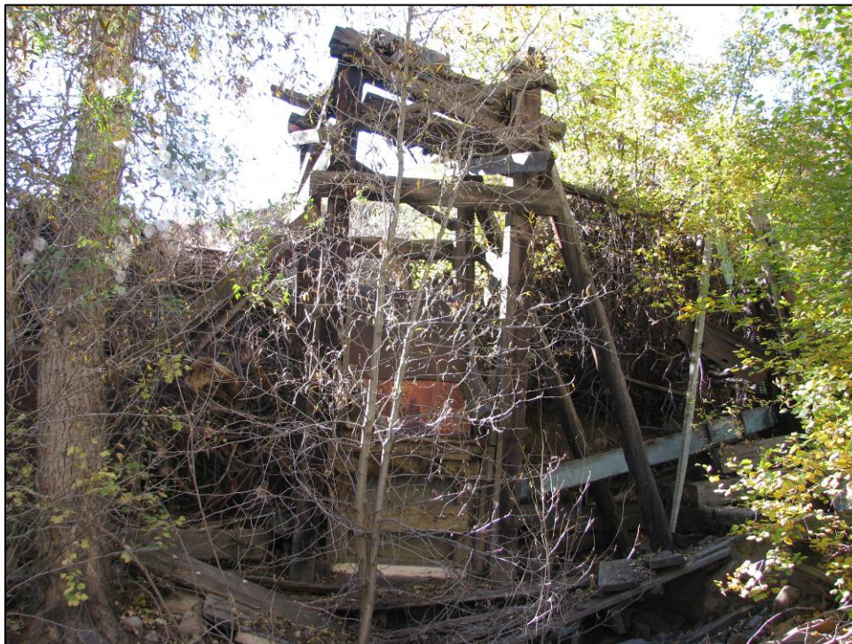
Figure 28. View south-southeast of the head frame at site 5CC1997, taken from the bank of Clear Creek.
