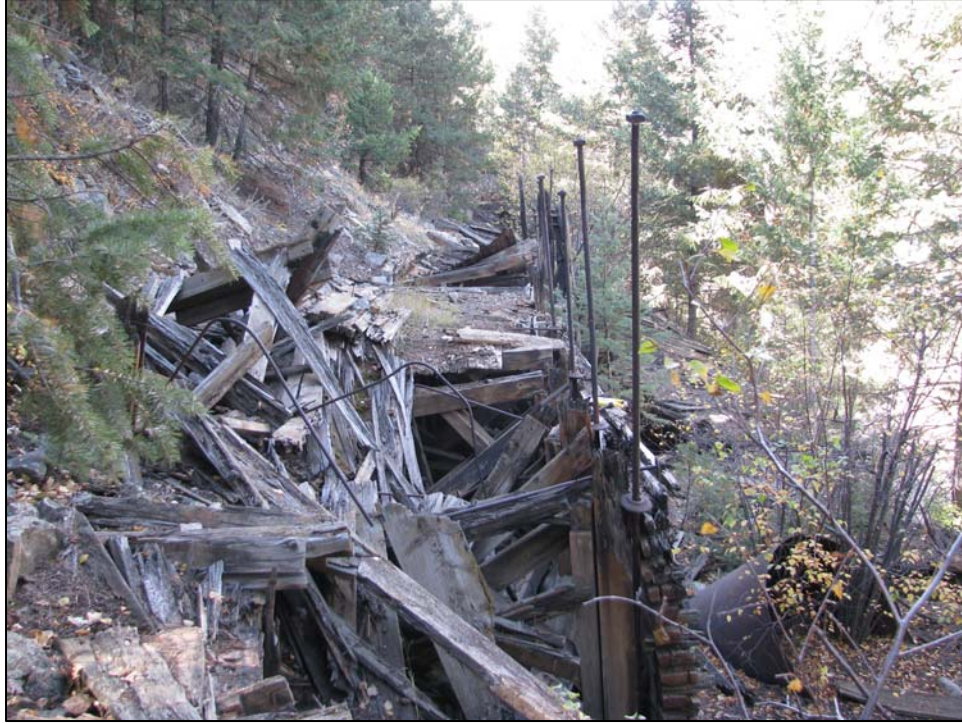
Figure 26. View east of the flume support structure and the remains of the water intake structure at site 5CC1996, with a short section of the conduit pipe at the bottom right of the photograph.
