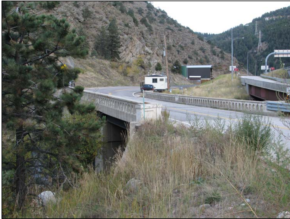
Figure 11. View southeast of U.S. Highway 6/40 segment, site 5CC2002.2. The bridge is site 5CC1078.
