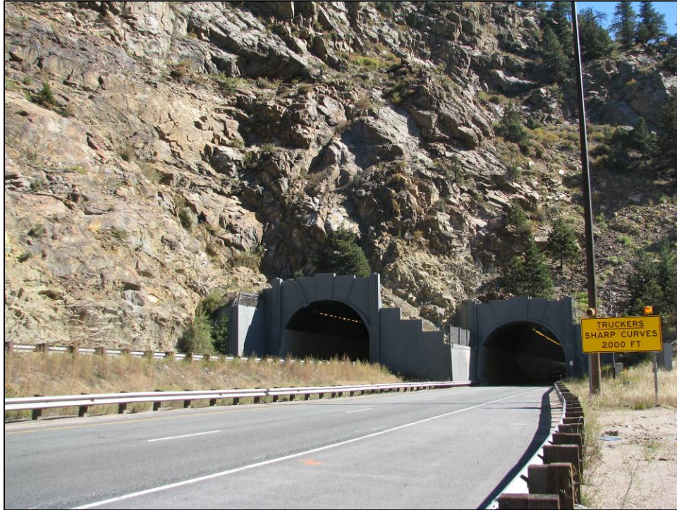
Figure 15. View of the west portals of the Interstate 70 Twin Tunnels, site 5CC1189.3, facing northeast.
