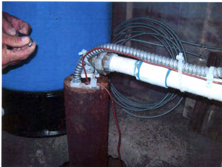
Attachment # 6 - Well 004: Due to the extent of the corrosion/deterioration the system should closely monitor this well head.
