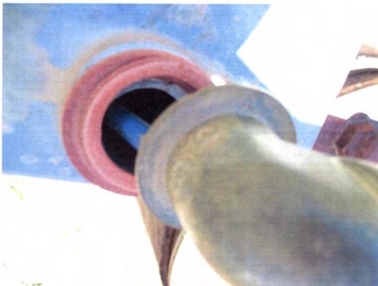
Attachment # 4 - Well 005: Electrical conduit box is detached.
