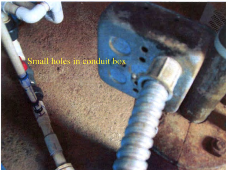
Attachment # 2 - Well 003: Small pre-drilled holes in the electrical conduit box.
