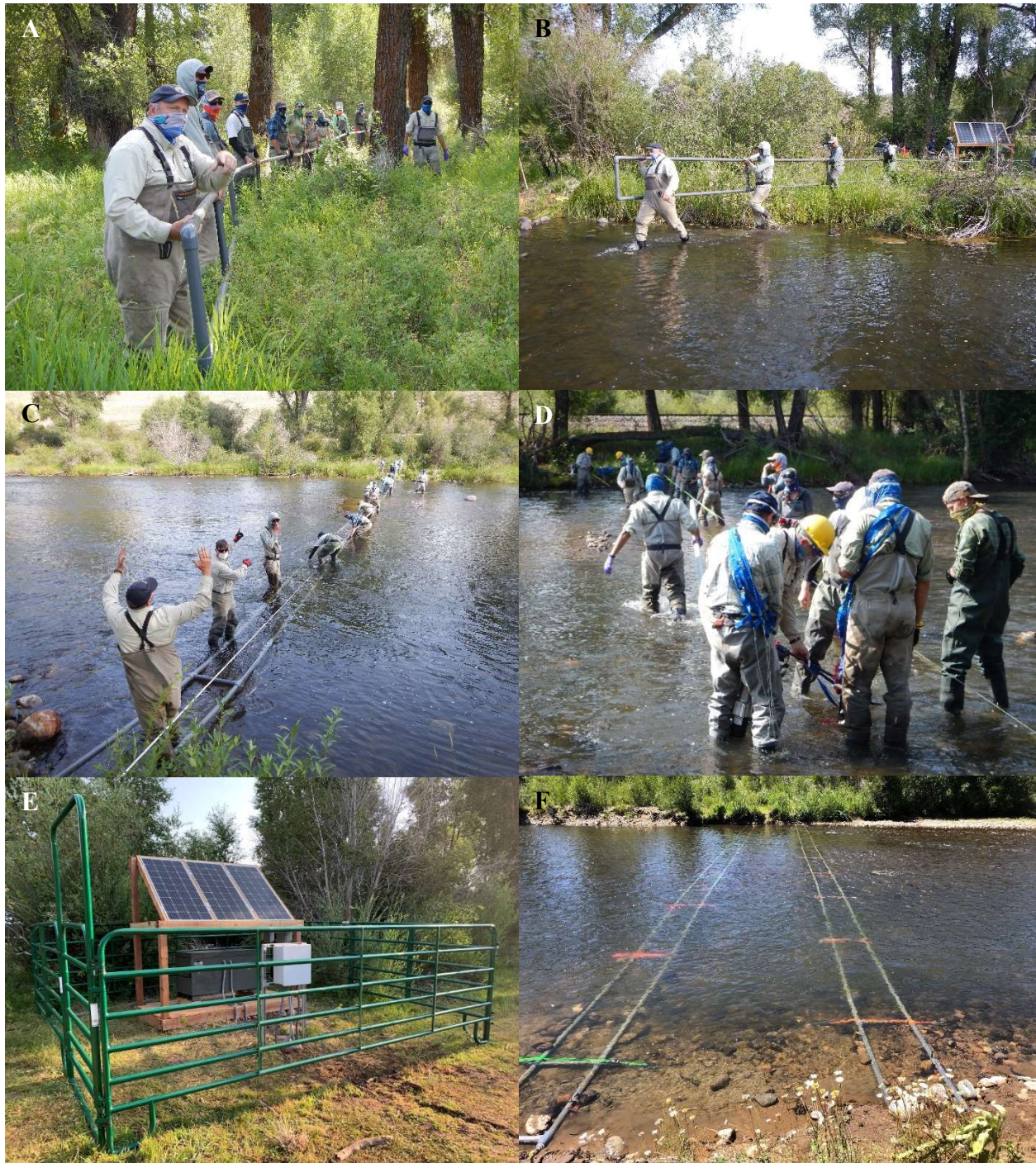
Figure 2.10. Antenna crews navigated the long, pre-made antennas through onshore obstacles (A), walked the antennas into the river (B), and placed them in the trenches dug in the substrate (C). Duckbill anchors were installed, and river and ratchet straps were used to hold the antennas in place (D). A cattle fence was also constructed around Red Barn to prevent damage (E). Two antennas were used to determine directionality of movement at each site (F).
