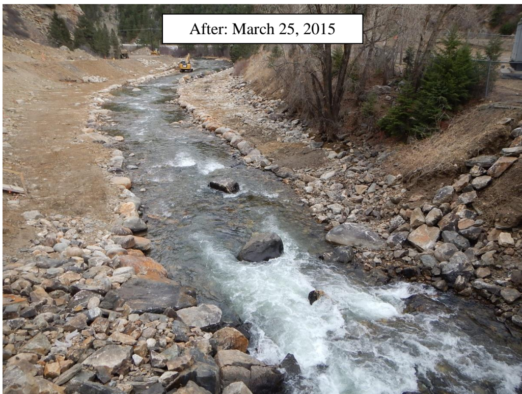
Figure 1.2. Post-construction photo of the moderately-confined “high-intensity” stream site as part of the Twin Tunnels project on Clear Creek.
