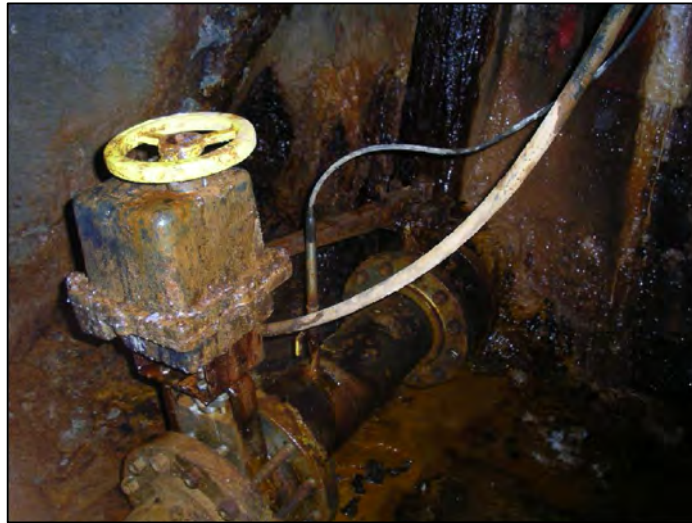
ELECTRONIC VALVE, TRANSDUCER AND MANUAL VALVE (2006)
