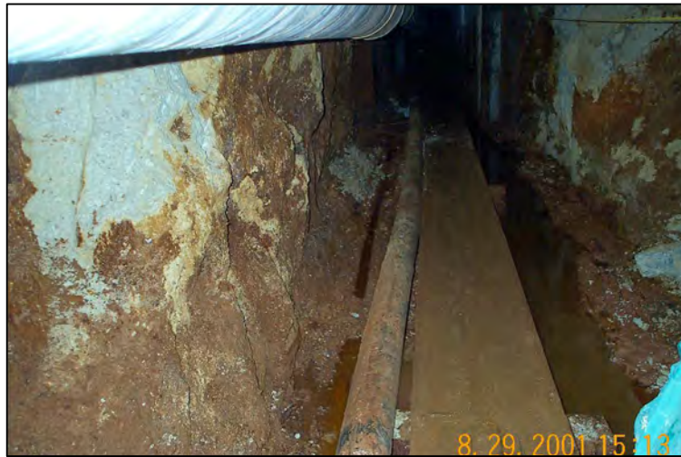
HDPE PIPE BETWEEN BULKHEAD AND STA 6+50 (2001)
