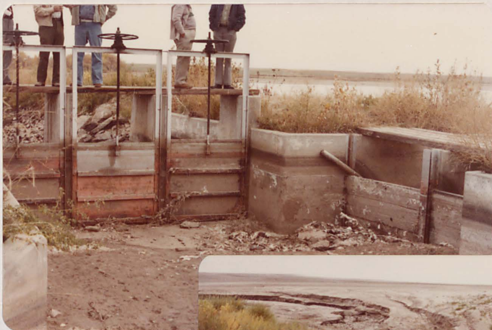
Lower diversion structure at Station 31+50 is in spillway reach as shown on Plate 5, Appendix D
