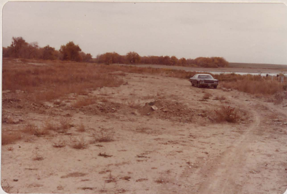
Spillway is about 1150 feet in length. Sandstone crest is about 950 feet wide. Elevation is 25.0 gage, 3.5 feet below crest of dike.
