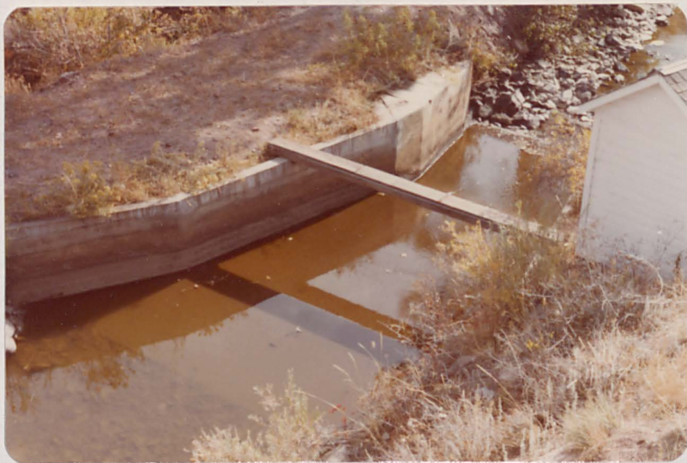
Parshall flume just below intake structure measures flow going to Lonetree Reservoir
