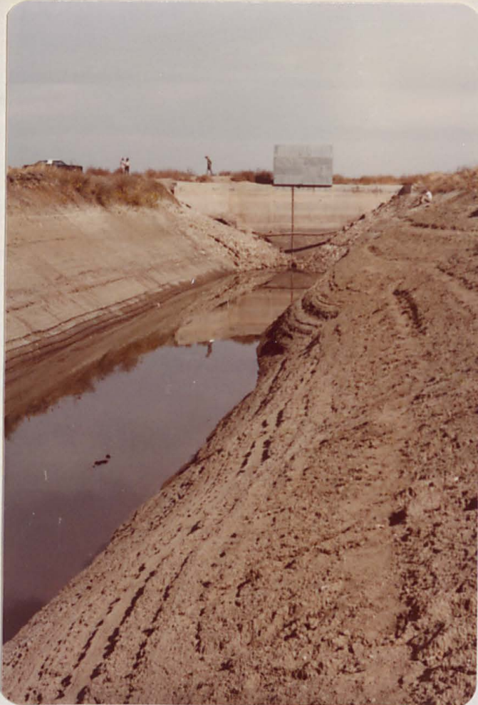
Concrete structure was placed against old masonry dam which is backed up with earth embankment as shown on Plate 2, Appendix C
