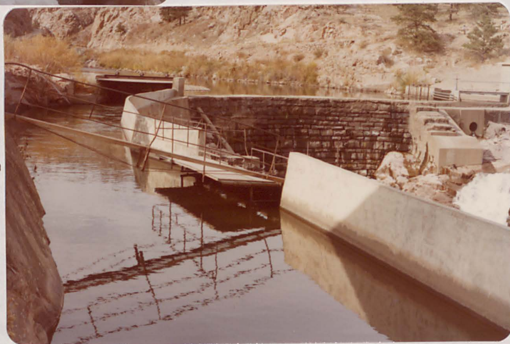
Intake for Home Supply Canal. Note wasteway back to river in foreground.
