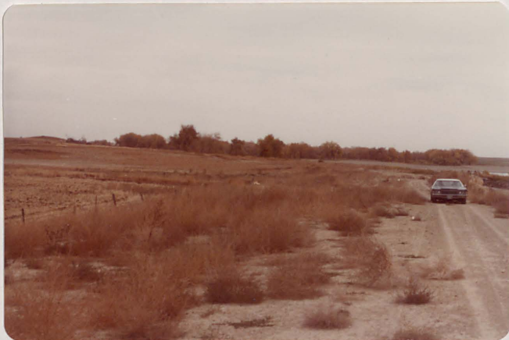
More distant view of spillway cut. Note swale to left of spillway. This is beginning of Ryan Gulch which would carry spill to Big Thompson River.
