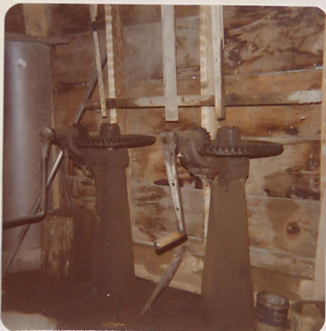
Gate hoists operate two 24" x 36" Armco slide gates
