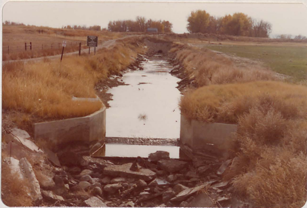
Downstream face of Lonetree Dam below metal gate house resting on top of dam in background. Parshall flume in foreground measures discharge from outlet into Lake Ditch Canal.
