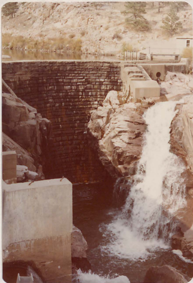
Masonry arch diversion dam supplies water to Home Supply Canal from right side of river. Structure withstood the 1965 flood.
