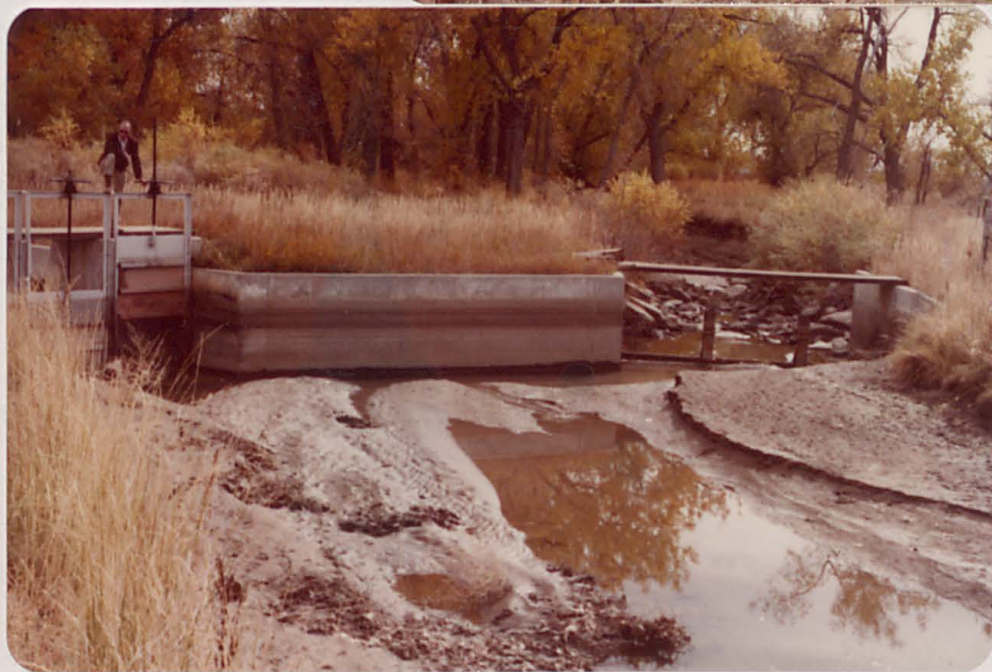
Upper diversion structure at Station 51+50. This diversion will handle 200 cfs. The supply canal can carry 350 cfs. When it does both diversion structures are used to fill the reservoir.
