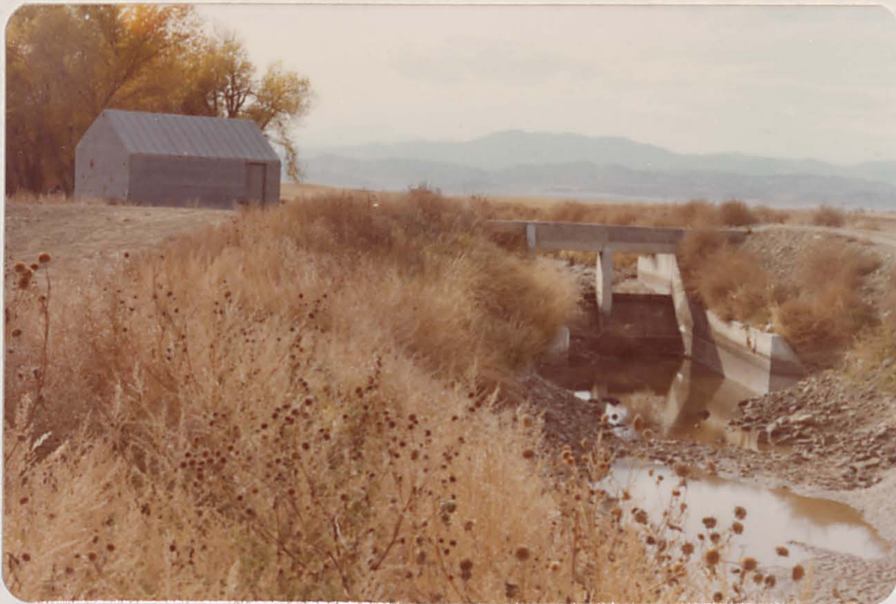
Metal gate house sits on Lonetree Dam. Outlet from dam to Lake Ditch Canal runs under Home Supply Canal. Crest of dam runs from barrier wall on top of check structure to contour 28.5 on right abutment.
