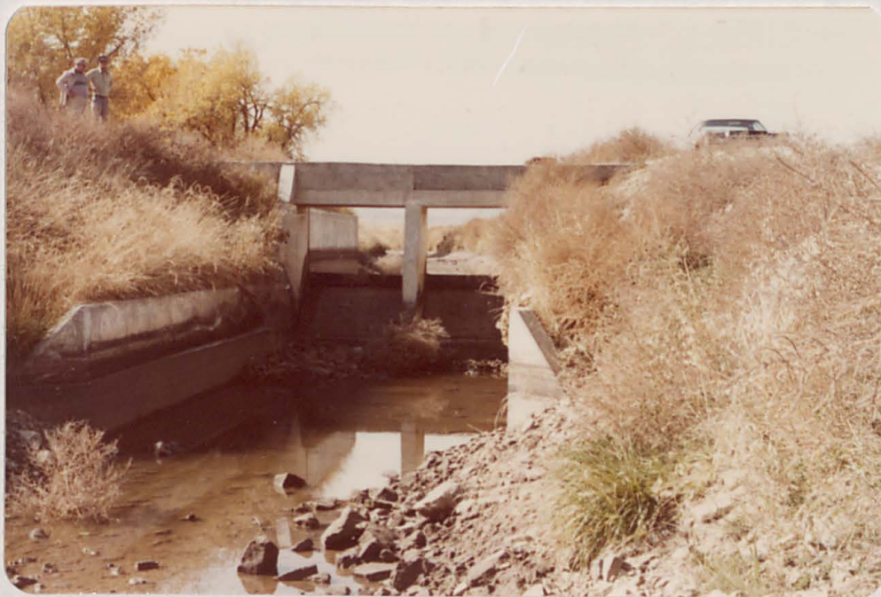
Concrete barrier wall was added to check structure to retain water spilling from Lonetree Reservoir into the Home Supply Canal. The barrier is 3.5 feet above spillway crest.
