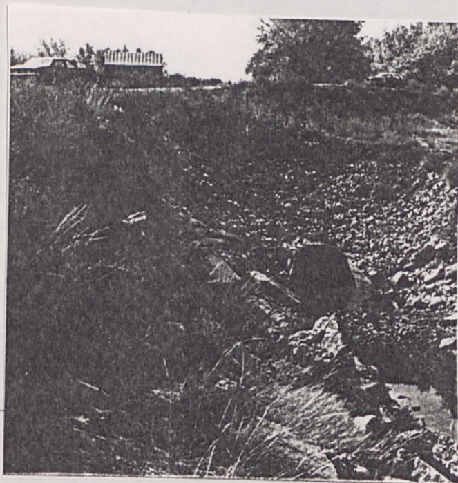
New seven-foot-long aluminum transition attached to a 60-foot-long, five-foot-diameter 14-gauge corrugated aluminum pipe extension to old 140-foot-long masonry arch tunnel
