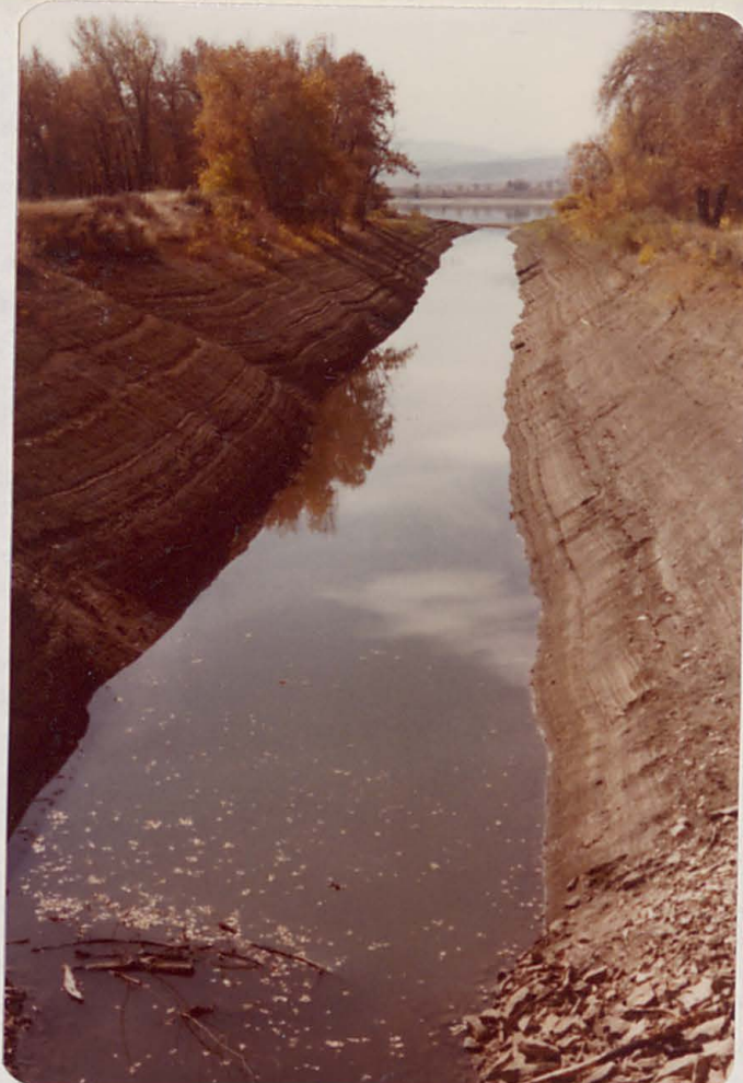
Looking upstream from top of dam. Intake structure is under water near branches in foreground.
