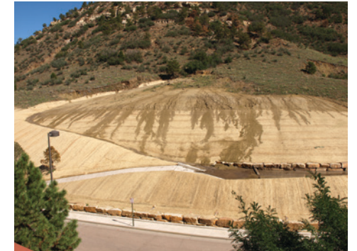
This relatively large landslide (slump) is moving ever so slowly downhill – the photo is taken from the roof of Monarch House
