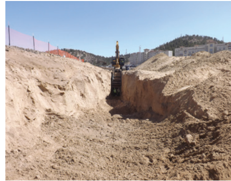
Excavation showing the sand dune at the construction site of the parking garage
