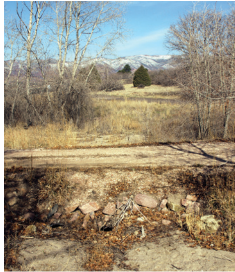
The culvert going below the road is almost completely blocked with sediment
