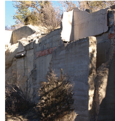
The remaining foundation of the 1930 nurses' quarters destroyed by expansive soils
