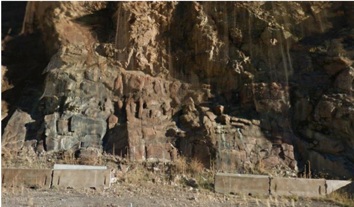
Photo 4. Example of Buttress and Sculpted Shotcrete on I-70 Corridor. Source: Google Earth 2015.
