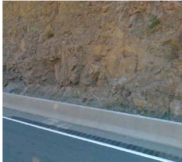
Photo 8. Example of a Type 7 barrier (to be replaced by Type 9 barrier)
