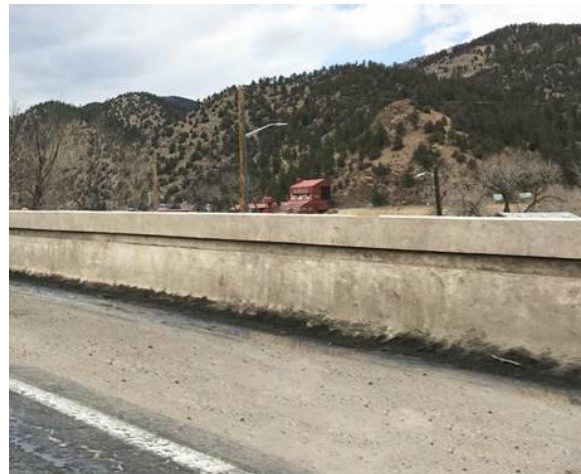
Photo 9. Example of a Type 7 barrier with glare screen (to be replaced by Type 9 Barrier with glare screen)
