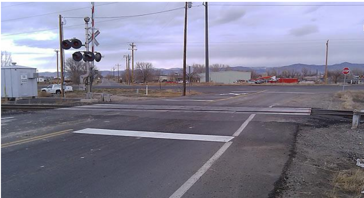
Intersection of 20 Road and Highway 6, looking north along 20 Rd. from south of RR tracks. Alignment of 20 Rd. north of highway can be seen running north into the distance. Misalignment of intersection can be seen in this photo.
