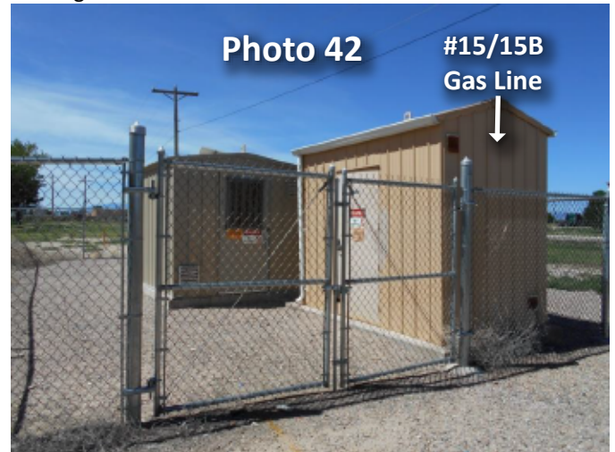
Two gas pipeline sheds are located on the west side of the Hewitt-Robin and Gartner USA building (GeoSearch Site 15/15B).
