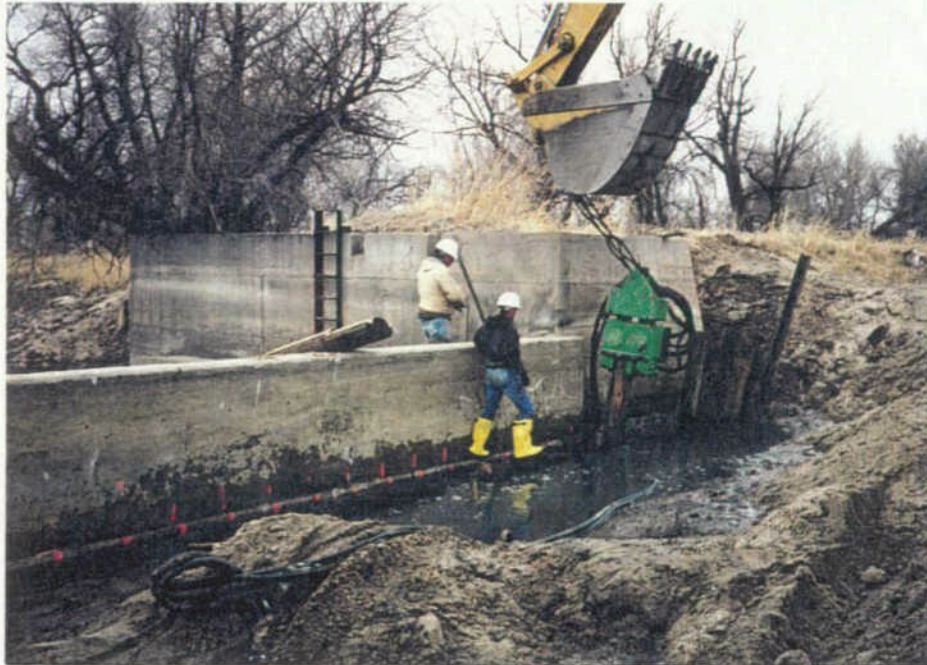
Placement of the Sheet Piling Along the Upstream Face of the Diversion Structure
