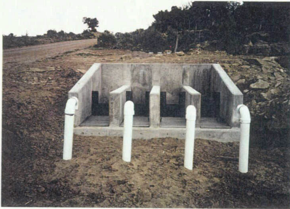
Looking toward the Multa Trina Ditch at the New 4-bay Concrete Division Box
