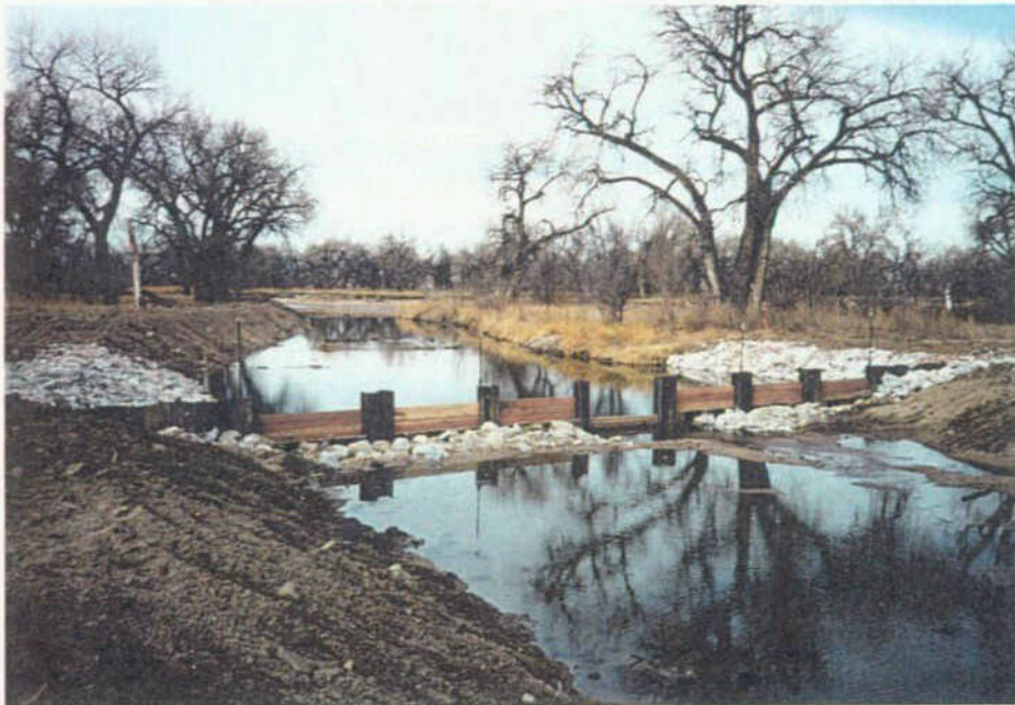
Looking D/S at the Check Dam Along the Side-Channel West of the Main Channel Diversion
