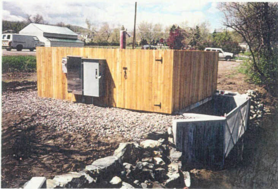
The Agricultural Ditch Pump Station at Colfax Avenue and Orchard Drive
