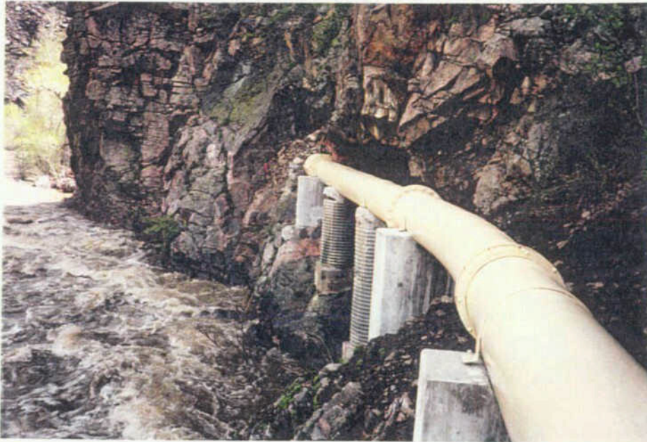
The 16" HDPE Transmission Line Encased in a 22" Steel Pipe Suspended Above Bear Creek
