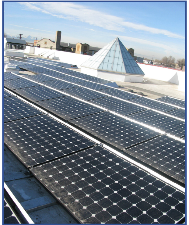
The solar photovoltaic system at the Brighton Library
