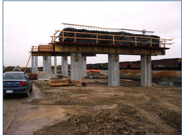
Construction of an overpass in Mesa County was made possible through funding created by SB09-232. This project is one of four that received substantial capital improvement dollars.
