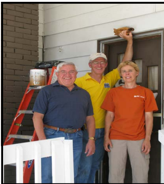
Checking on efforts at the Habitat for Humanity's "A Brush With Kindness" are Loveland Mayor Cecil Gutierrez, Gale (Counselor in LDS Loveland Stake Presidency), and Shelly, Construction Supervisor for "A Brush of Kindness".
