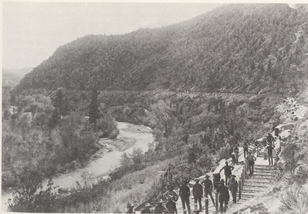
Figure 22. U. S. Gold Placer flume under construction about 1888, San Miguel River, Montrose County. (Denver Public Library, Western History Department)
