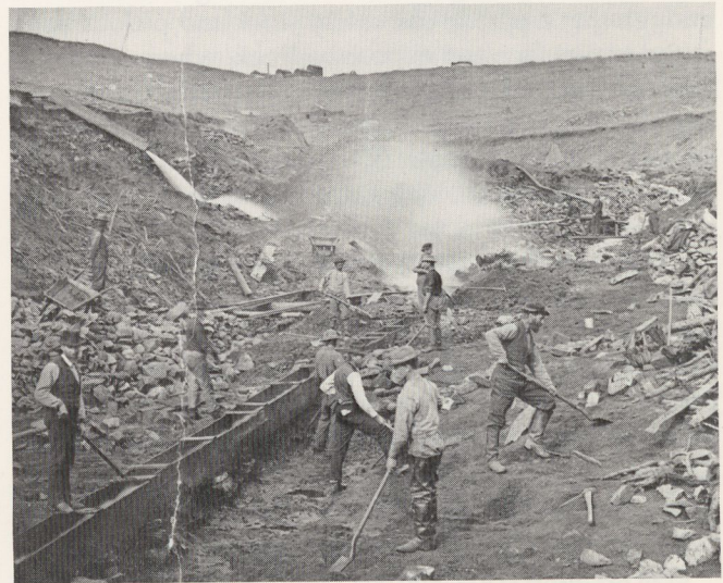
Figure 11. Miners are cleaning to bedrock in Illinois Gulch, Gilpin County—shoveling into the sluice the gravel originally resting on bedrock and any sand remaining from the sorting of gravel once lying higher above and now removed. The men are using the jet from a monitor and a stream of water to loosen the gravel and wash it toward the sluice. (Colorado Historical Society)
